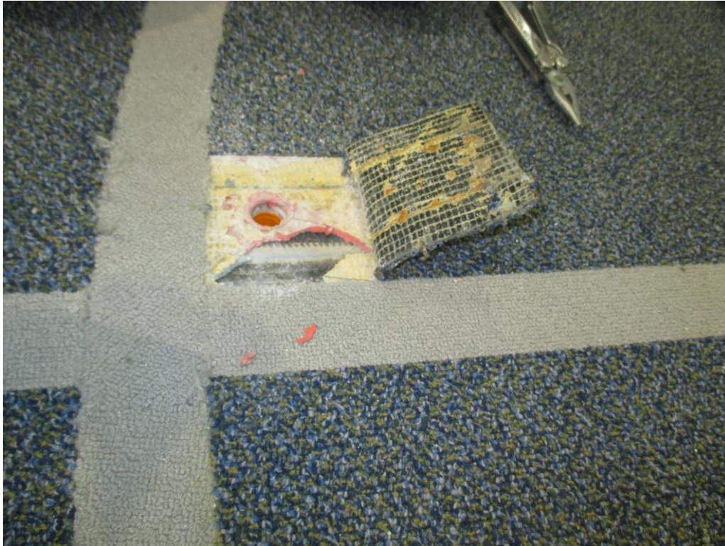
Photo 3 View of the orange center court tile under the carpet in the gym that is positive for asbestos.
