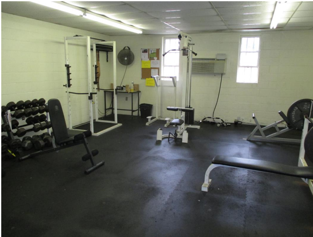
Photo 9 View across weight room. There are two layers of white floor tile located underneath the black rubber matting in the weight room. The bottom layer of floor tile is positive for asbestos.
