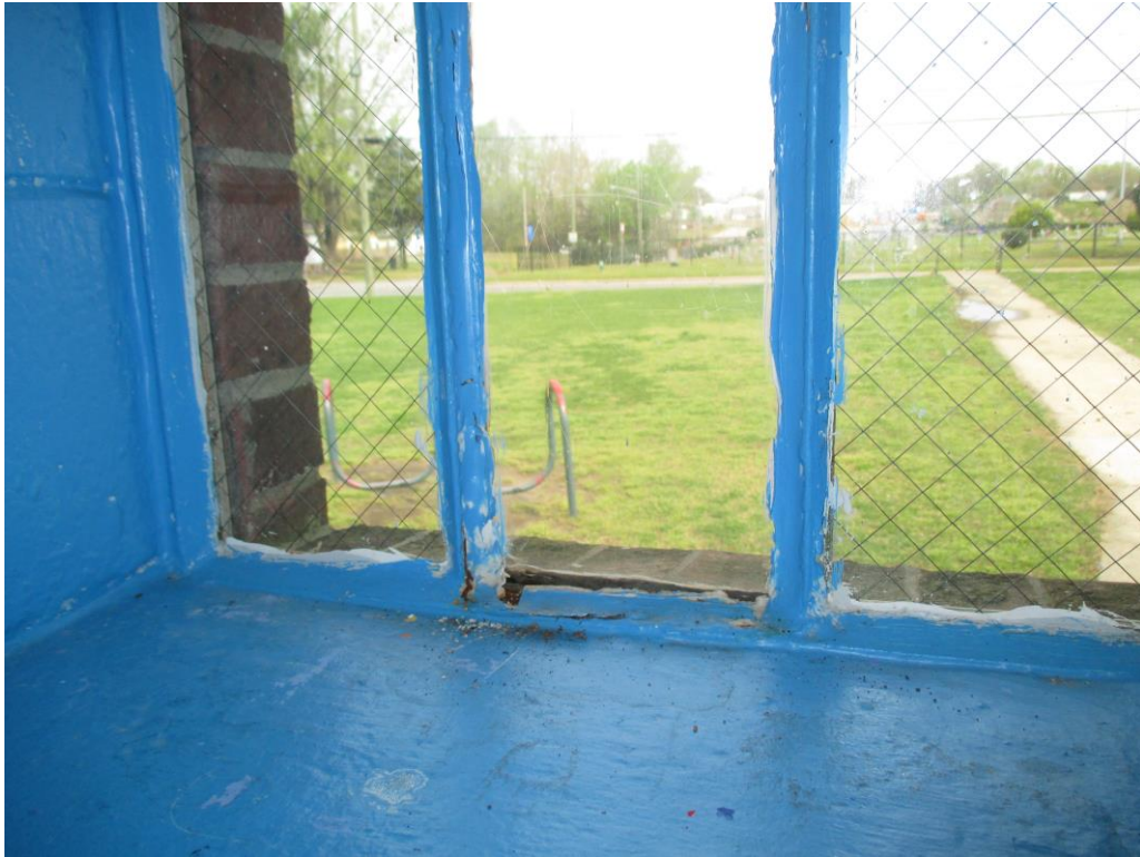
Photo 7 Close up view of the window frame. Showing window caulk and window glaze.
