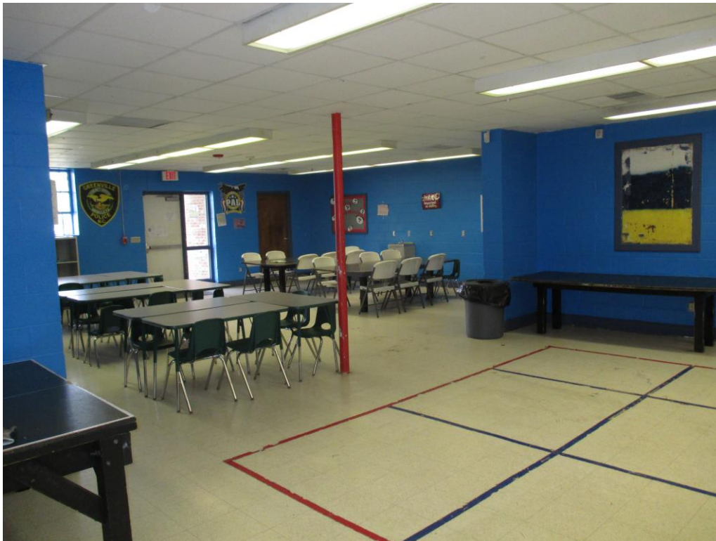
Photo 5 Typical view across the kid's area. Mastic under the floor tile in this area is positive for asbestos.
