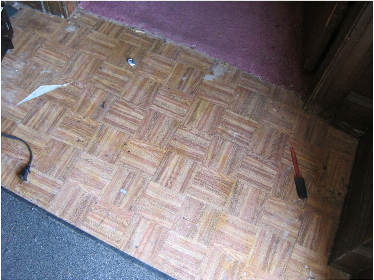
Vinyl flooring located in the side entry foyer of the church building.
