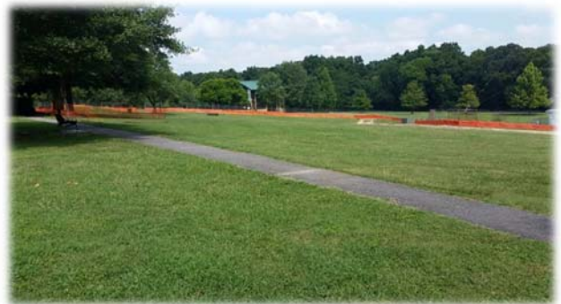
Fencing is in place to begin the construction for the inclusive playground.
