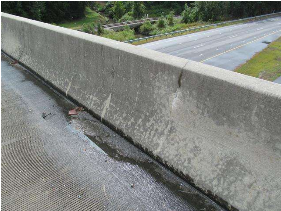
SIMILAR CRACKS AT RAILS.
