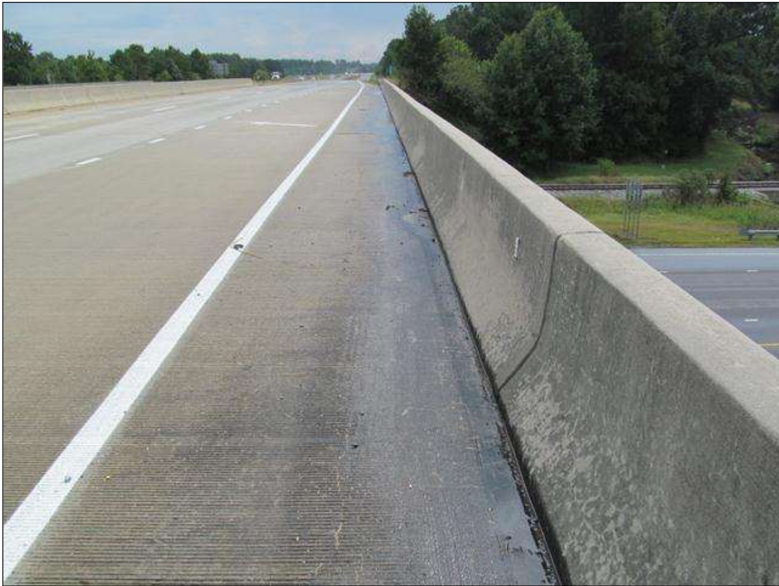
DEBRIS & PONDING ALONG RT RAIL. DEBRIS ALONG LT SIDE.
