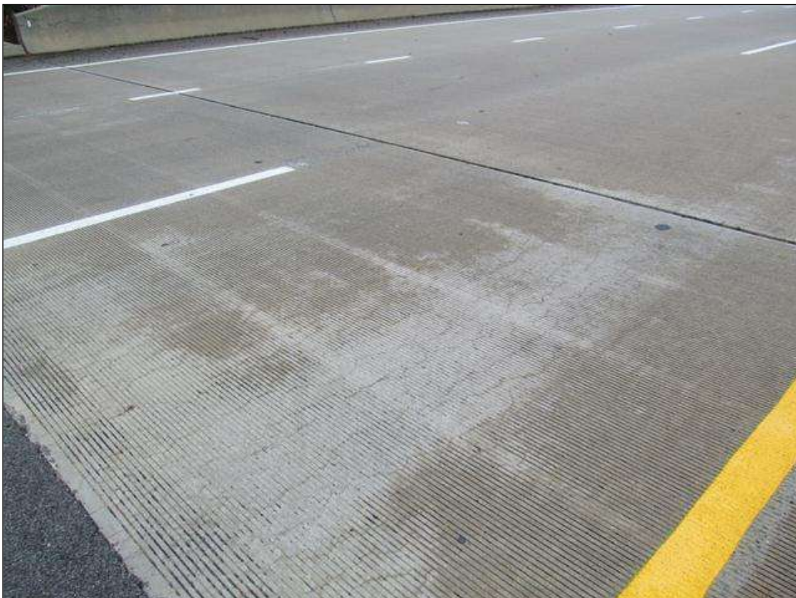
WEST APPROACH SLAB WITH CRACKS IN BOTH LANES. SIMILAR @ THE EAST APPROACH SLAB.
