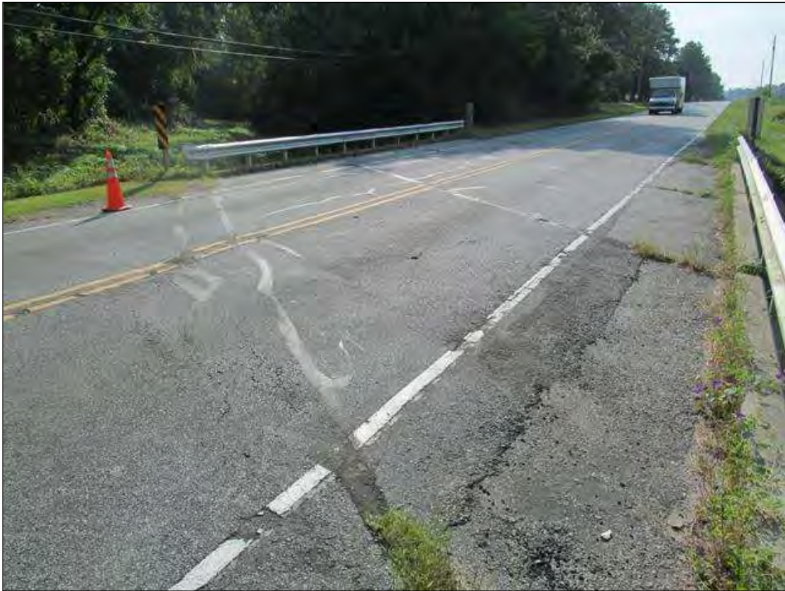
WEST APPROACH HAS UNEVEN TRANSITION. THE EAST END SIMILAR.
