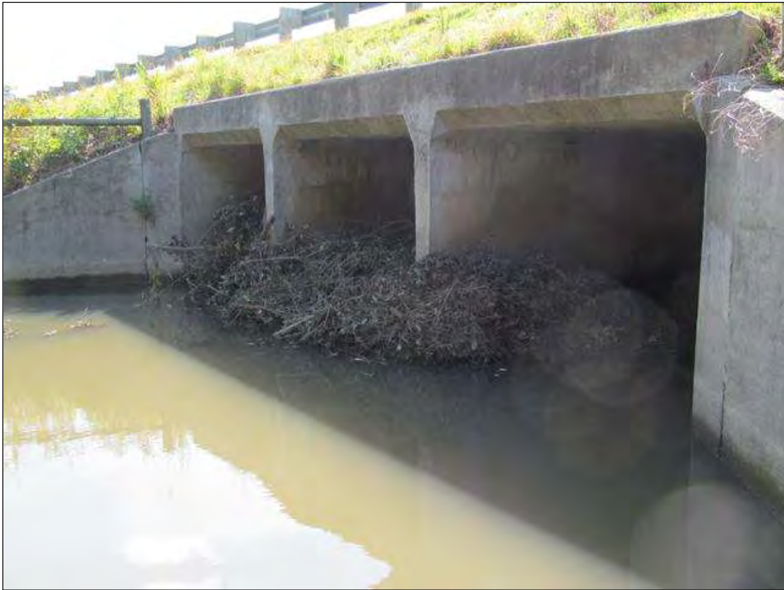
LARGE DRIFT PILE AT UPSTREAM END OF BARRELS.
