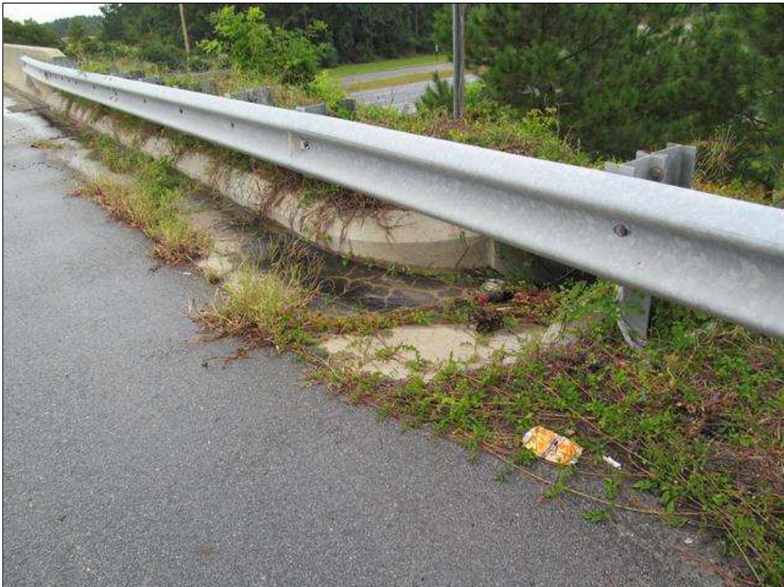
DEBRIS @ THE NE APPROACH DRAIN.
