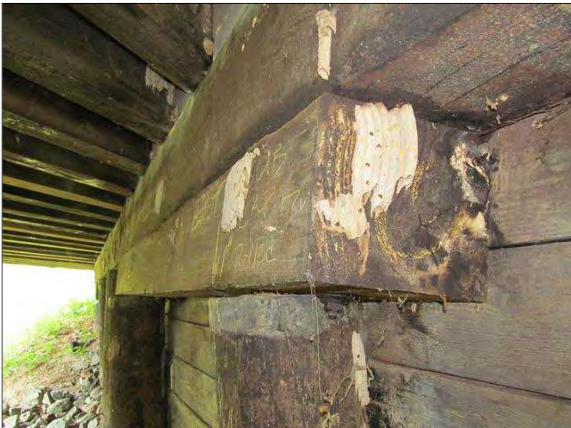
END BENT 1 SUBCAP #2 ROTATED WESTWARD WITH GAPS AT PILES. SUBCAP #1 SIMILAR AT END BT 1.
