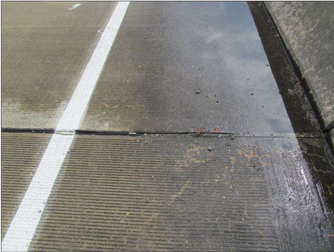
SIMILAR DEBRIS AT COMPRESSION SEALS.
