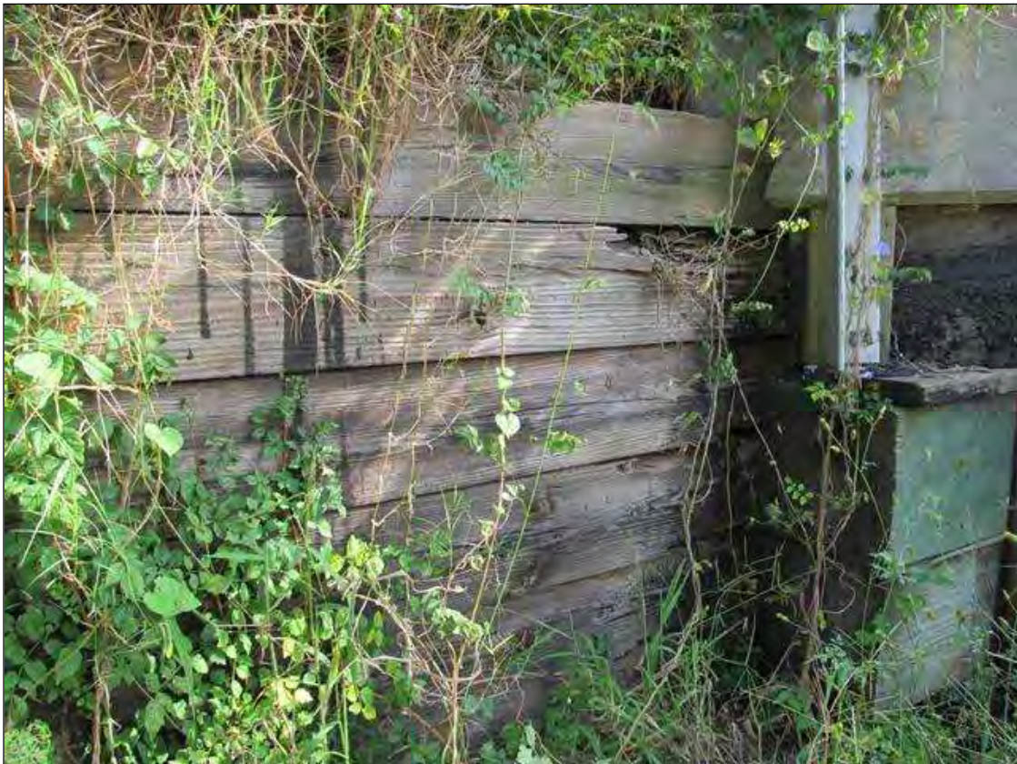
SW EXTERIOR BULKHEAD HAS DECAYED BOARDS.
