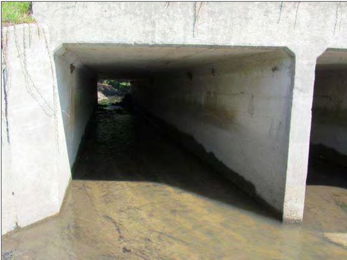
BARREL 1 IS PARTIALLY BLOCKED BY DRIFT WITH MAIN FLOW AT THIS LINE.
