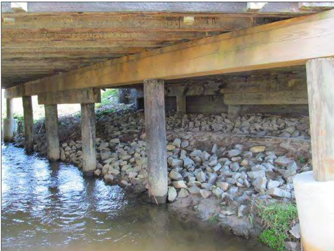
SPAN 2 SIDE OF BT 2. (P-1 & 6 HAVE TEMP. REPAIRS) (BT 1 SIMILAR WITH NO REPAIRS TO PILES.)
