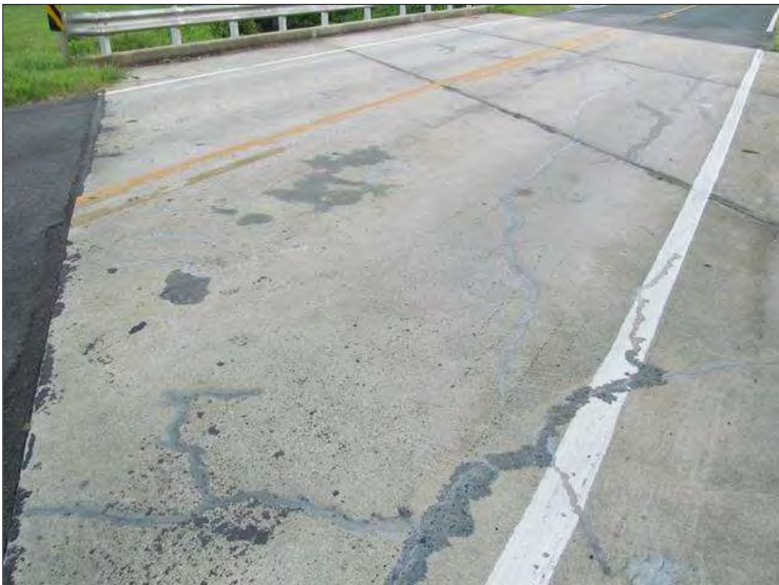
SPAN 1 DECK WITH SEALED CRACKS. SIMILAR IN SPANS 2 & 3.
