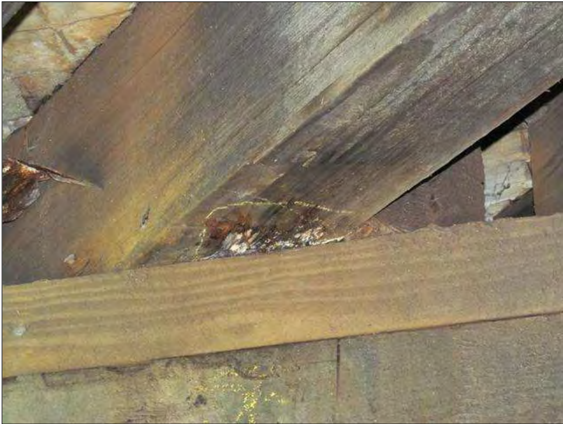
J-11 IN SPAN 1 DECAYED AT BEARING OVER BT 1
