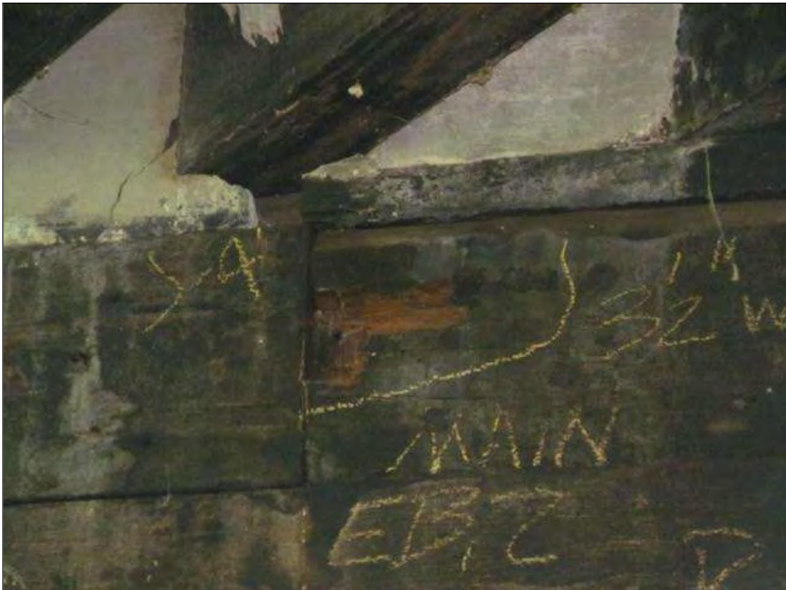
END BENT 2 MAIN CAP DECAYED AT SPLICE POINT #1 UNDER J-4.
