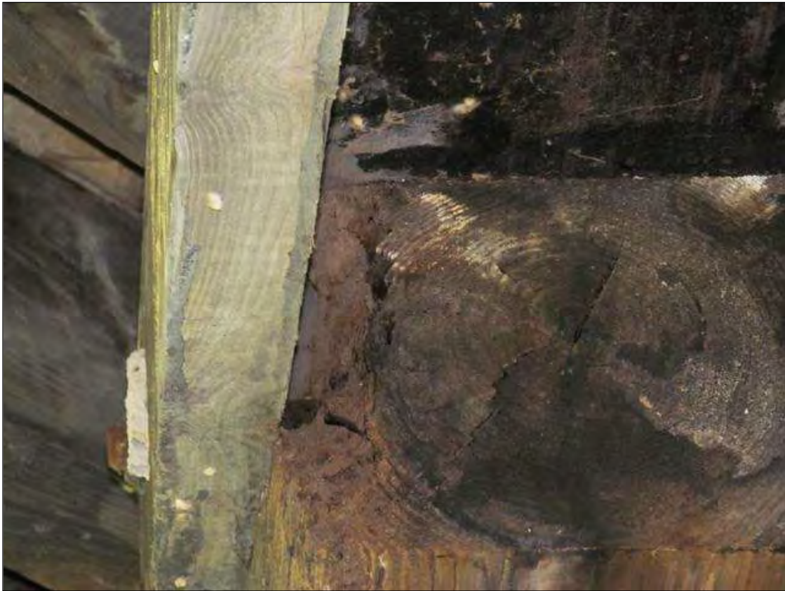
BENT 2 SUBCAP #2 DECAYED
