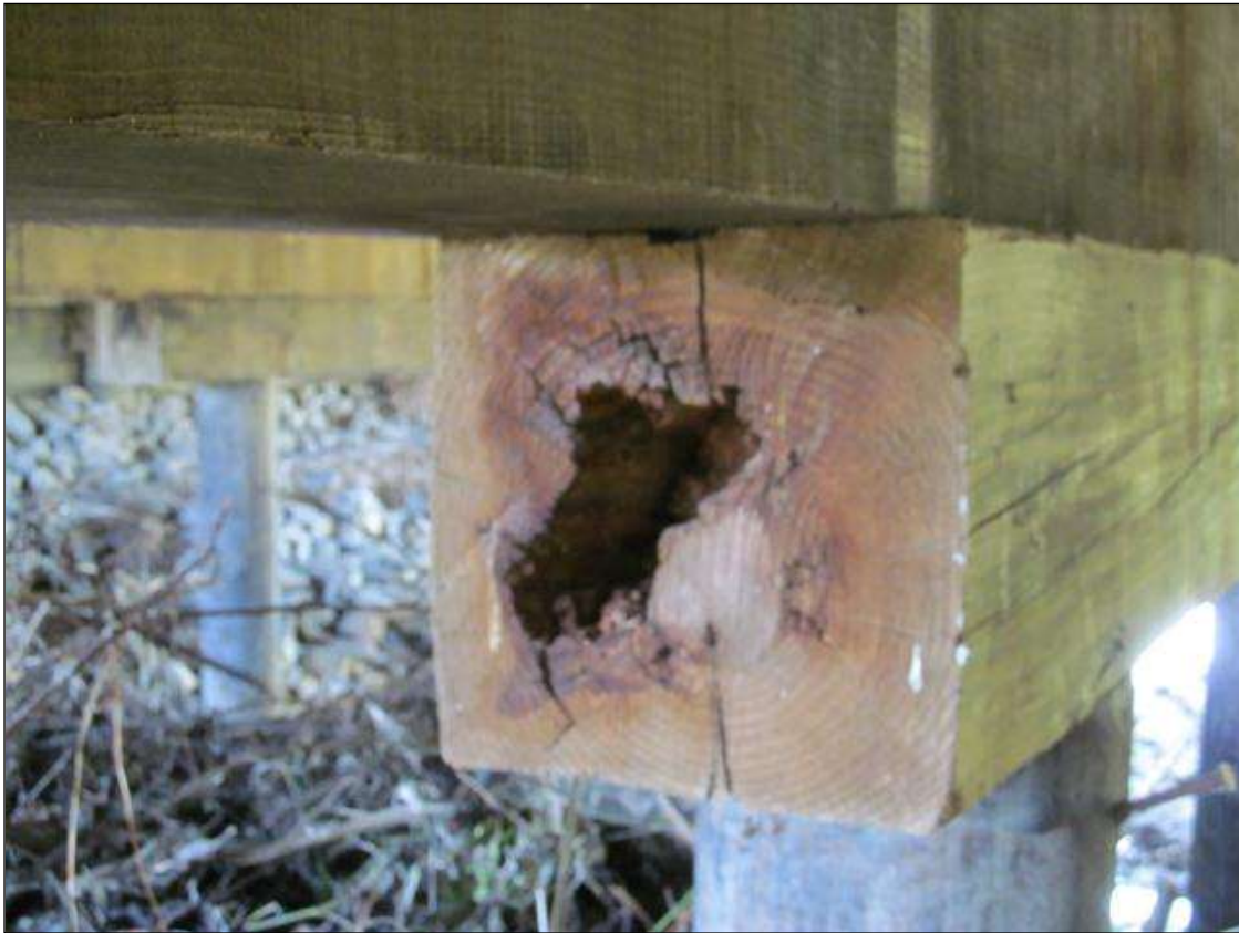
LT END OF BENT 1 SUBCAP DECAYED.
