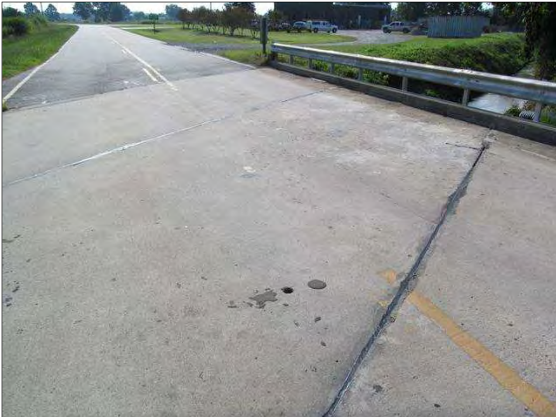
LONGITUDINAL CRACKS IN SPANS 2 & 3.
