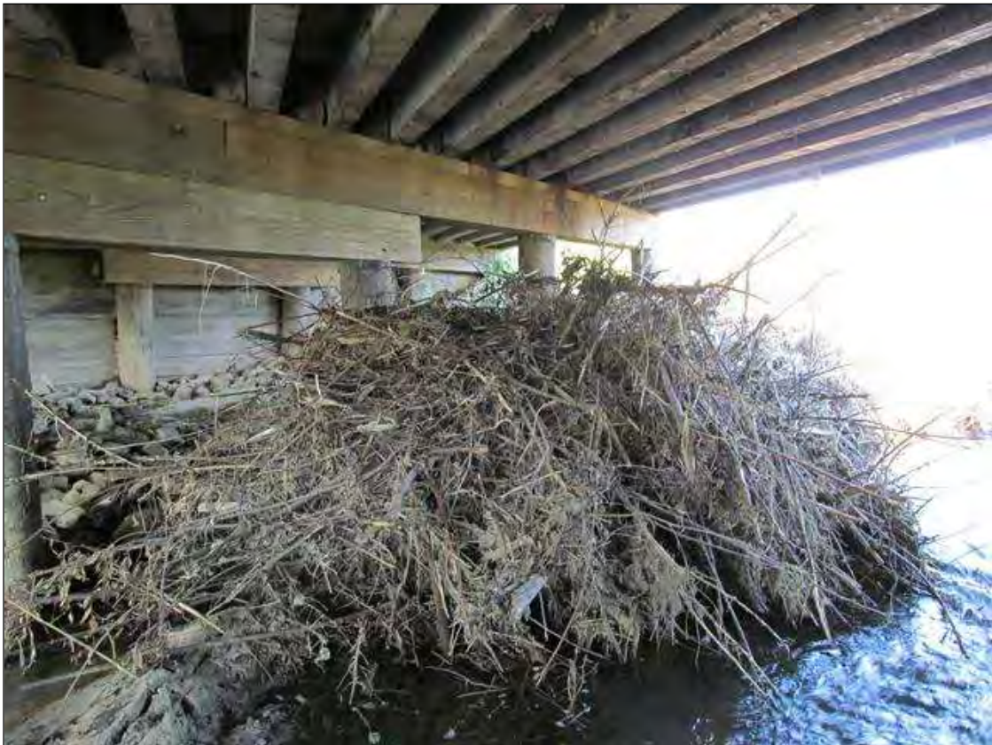
(PM)-LARGE DRIFT PILE AT SPAN 2 SIDE OF BENT 1.
