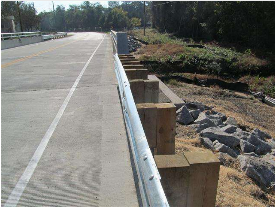
SW GUARDRAIL POST SPACINGS @ THE TRANSITION. SIMILAR @ ALL CORNERS.
