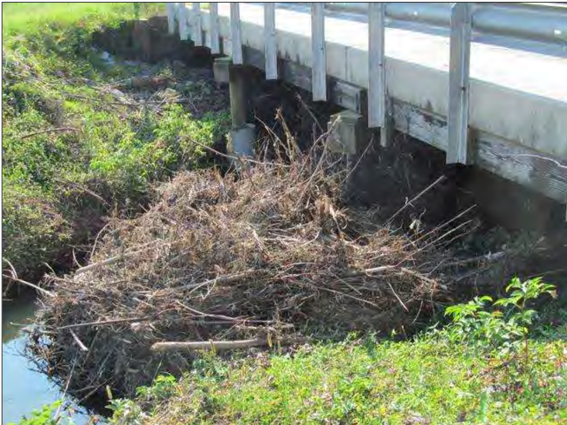
(PM)-LARGE DRIFT PILE AT SPAN 1, BT 1 & SPAN 2.
