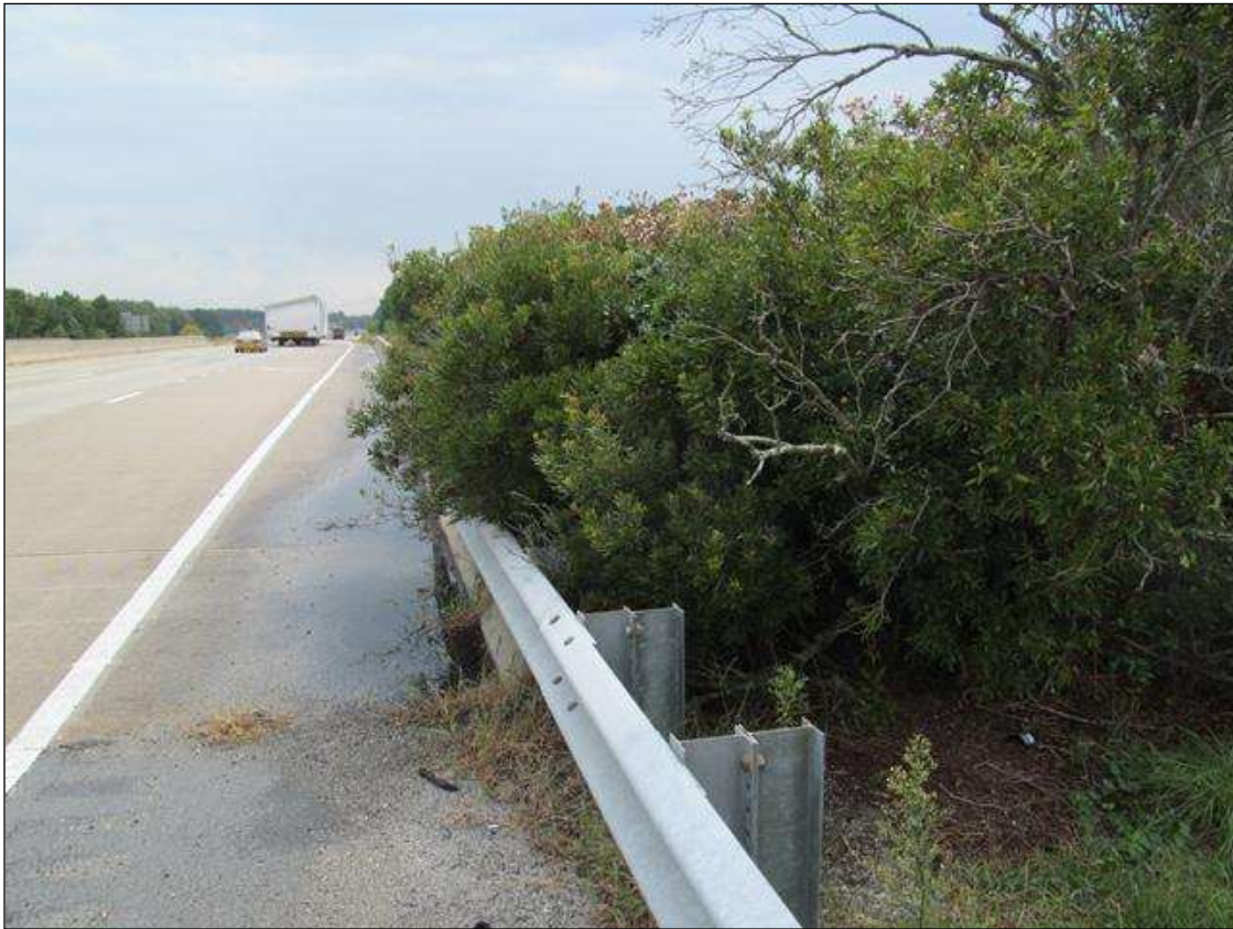
SHRUBS AT SW SLOPE OVERTAKING GUARDRAIL.
