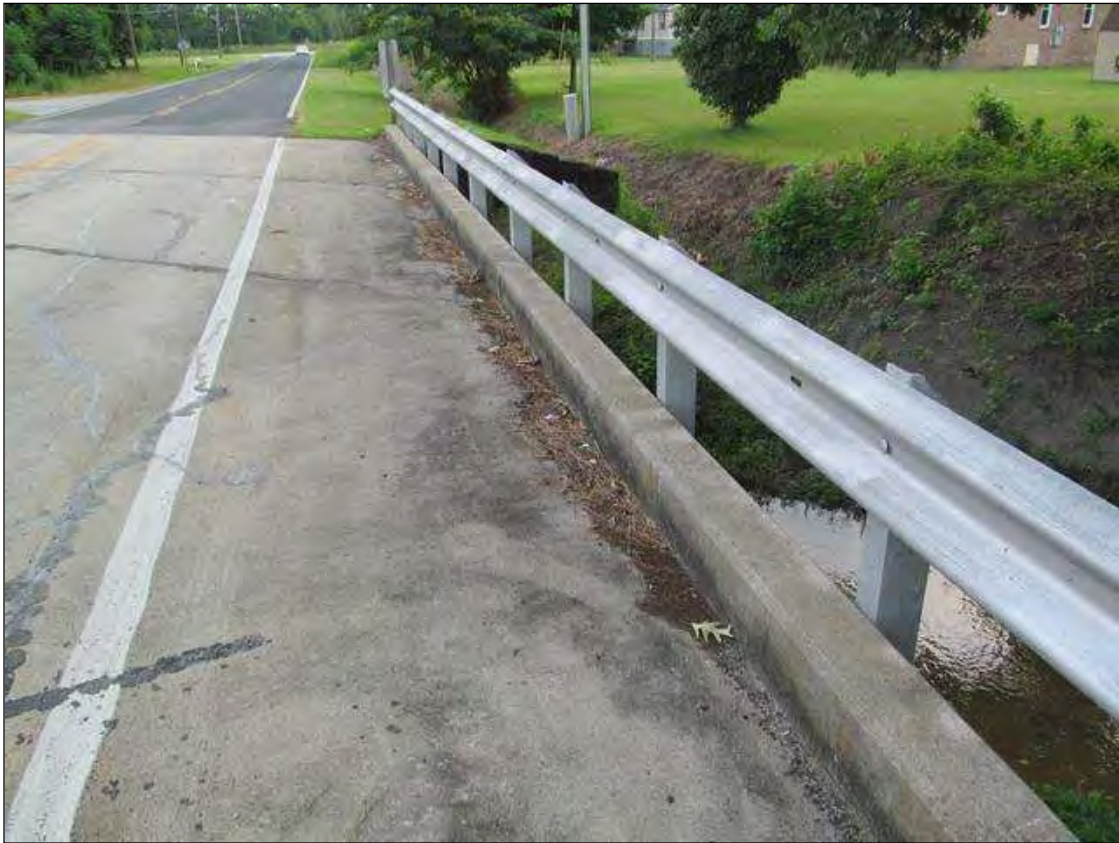
DEBRIS ALONG THE RIGHT CURB WITH BLOCKED DRAINS. SIMILAR ALONG THE LEFT CURB.
