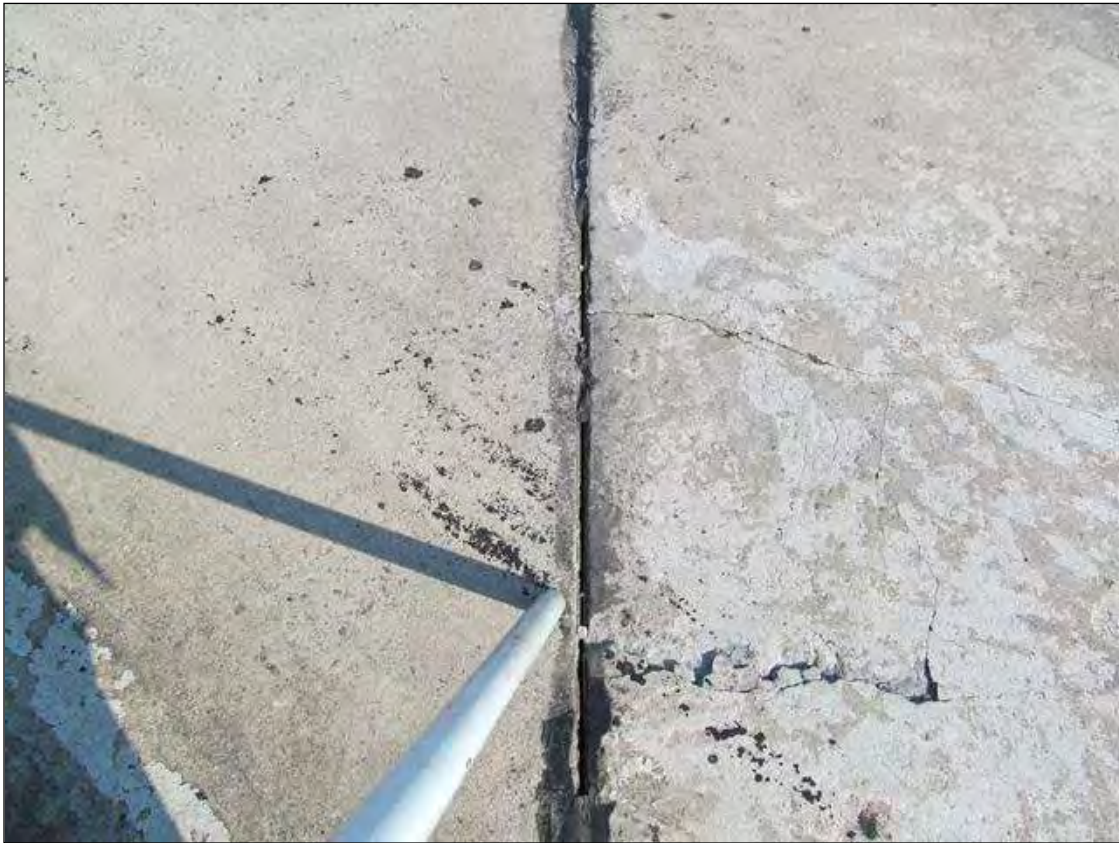
JOINT MATERIAL MISSING AT BT 1, RT LANE.
