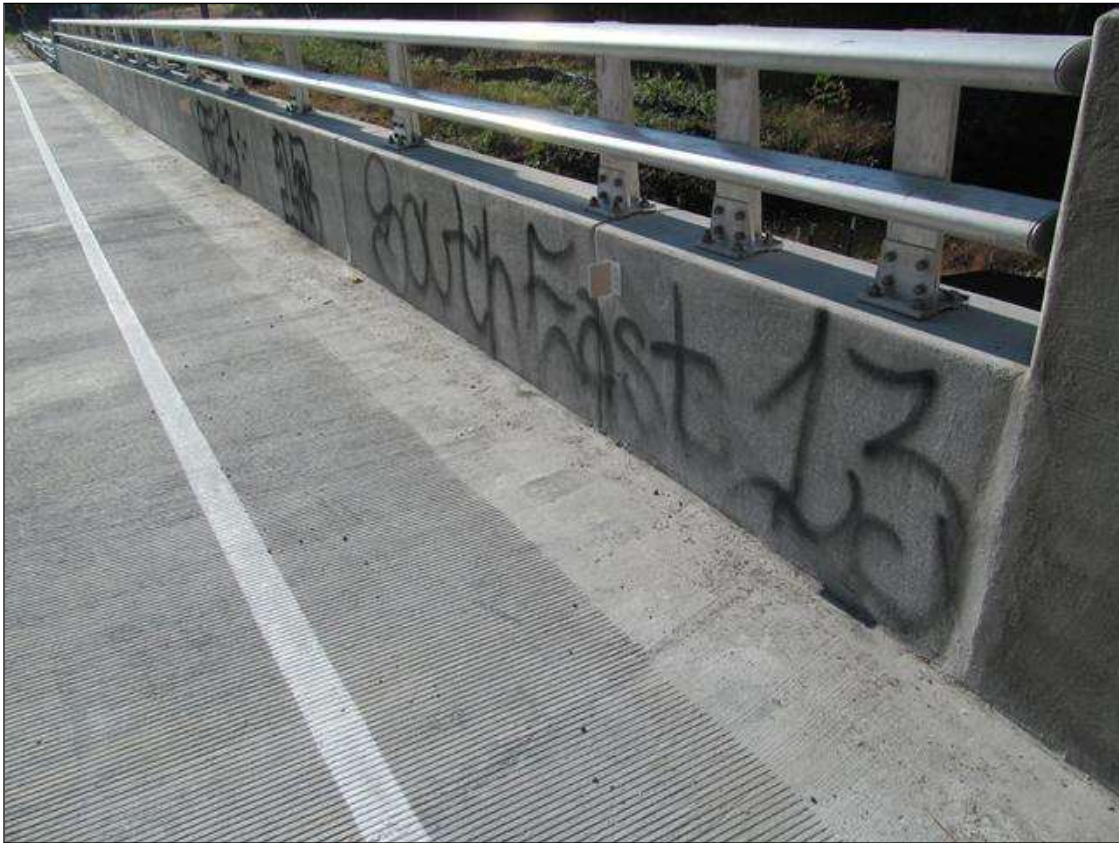
GRAFFITI ALONG THE RIGHT PARAPET.
