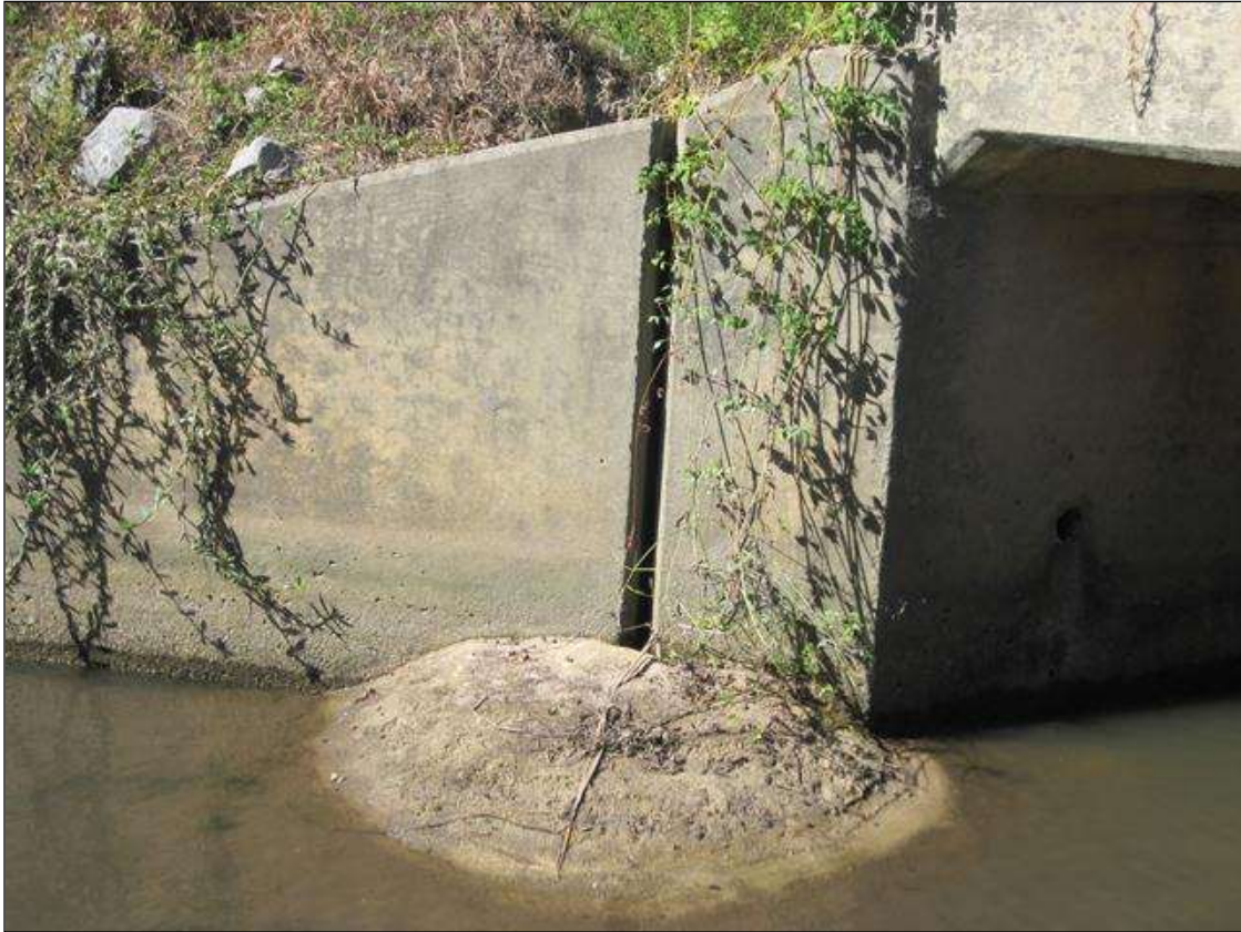
MISSING EXPANSION JOINT MATERIAL AT SOUTHWEST WINGWALL WITH FILL FILTERING THROUGH
