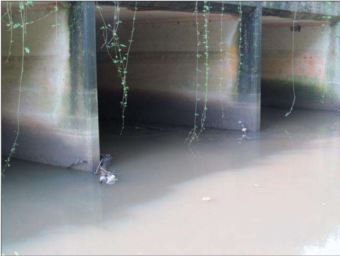
DRIFT @ THE NORTH END OF THE INTERIOR WALLS.
