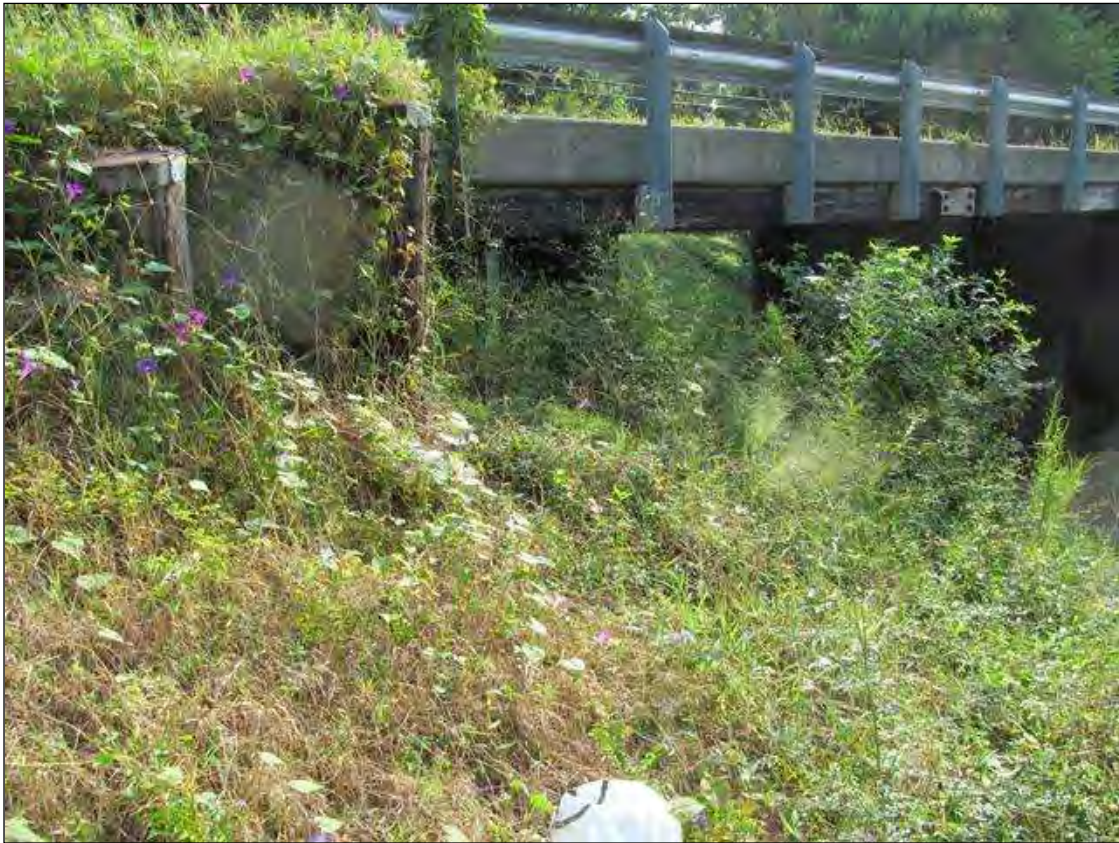
VEGETATION AT SW SLOPE. SIMILAR AT ALL CORNERS.
