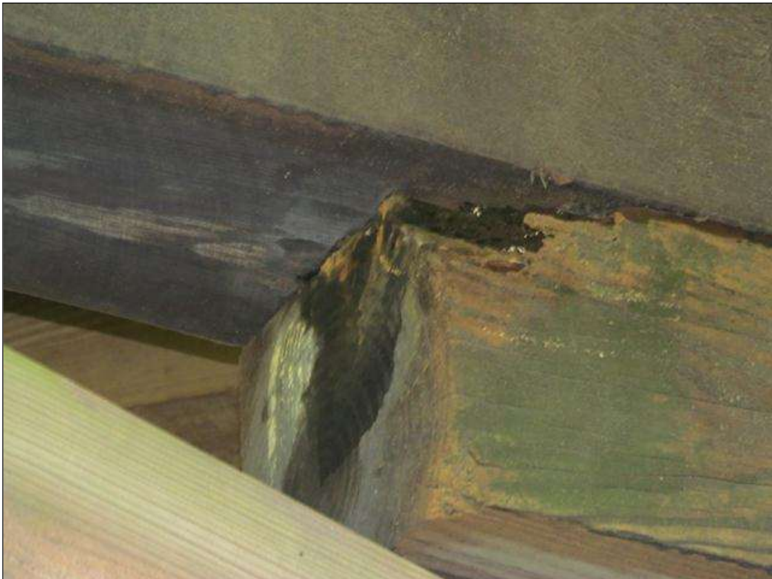
BENT 1 SUBCAP #2 DECAYED
