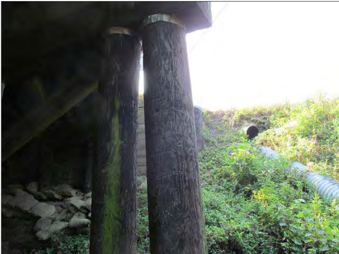
P-9 AT BENT 2 DELAMINATED AND SOUNDS HOLLOW BEHIND THICK FACIAL SHELL.
