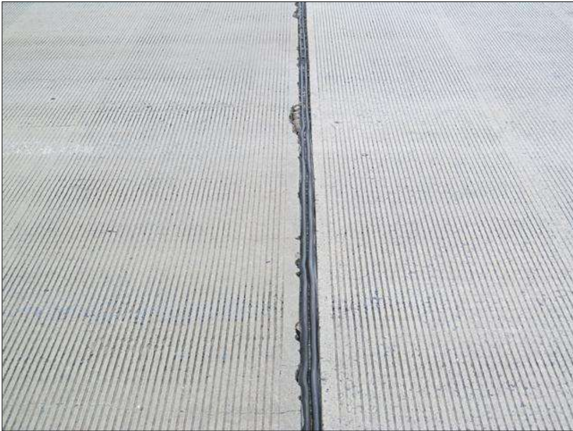
COMPRESSION SEAL @ EBT.2 WITH SEPARATION & DEBRIS ALONG THE JOINT. OTHERS ARE SIMILAR.
