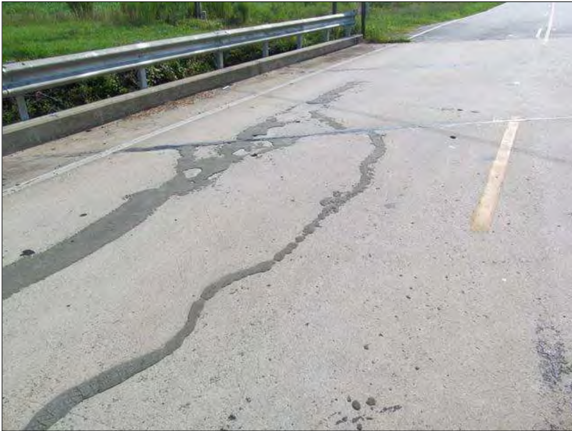
SIMILAR DECK WITH CRACKS AND PORTIONS SEALED IN LT LANE OF SPANS 1 & 2. OTHERS NOT SEALED IN RT LANES IN SPANS 2 & 3.
