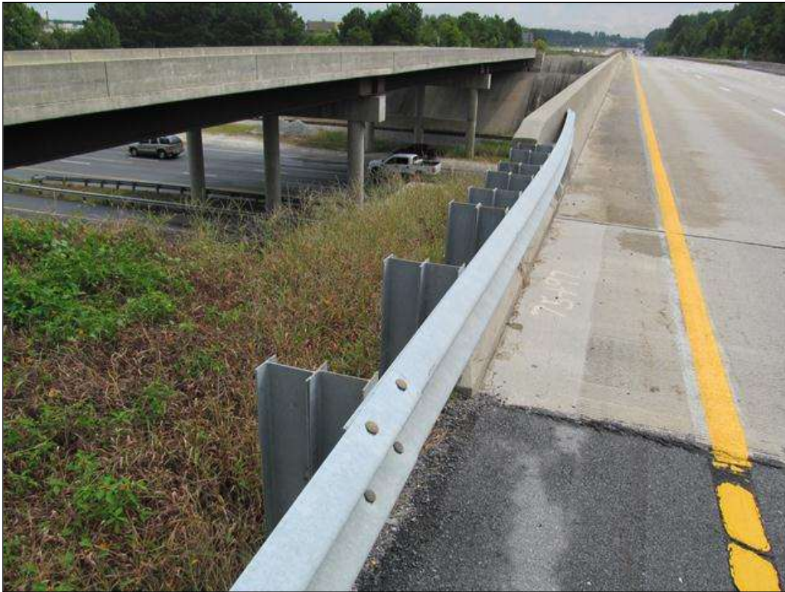
NW GUARDRAIL POST SPACINGS AT TRANSITION TO BRIDGE RAIL. (SW TRANSITION SIMILAR)
