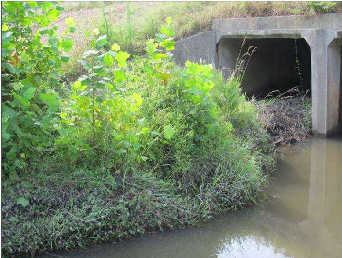
BARREL 2 BLOCKED WITH SILT & VEGETATION.
