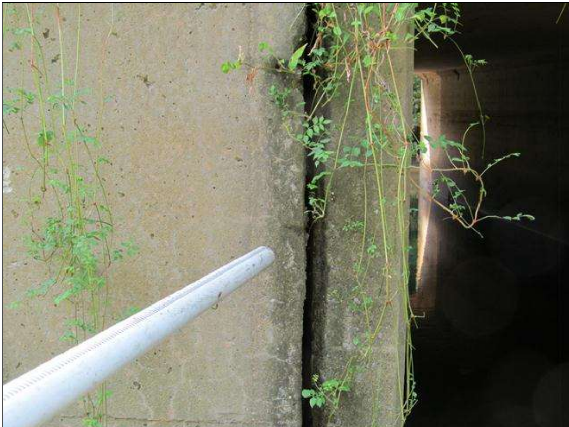
JOINT MATERIAL MISSING @ THE NE CORNER. SIMILAR @ ALL CORNERS.
