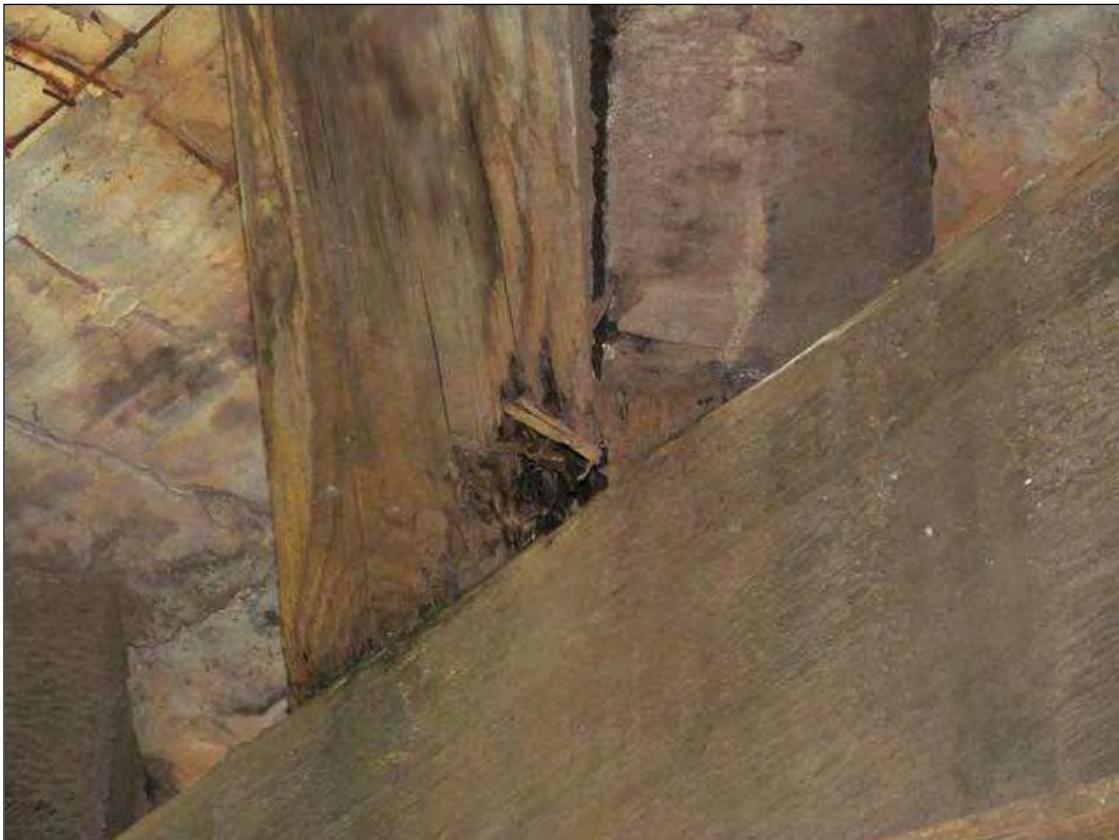
J-15 IN SPAN 2 DECAYED AT BEARING OVER BT 1
