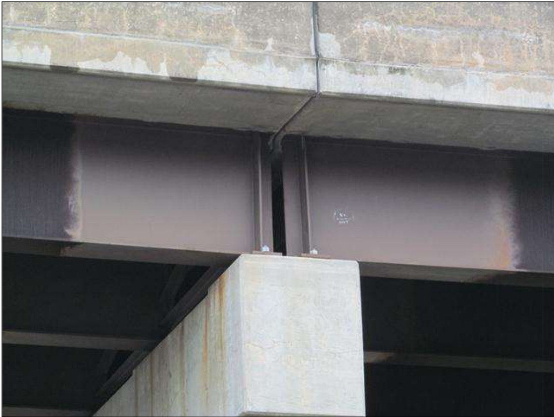
WEATHERING STL. BEAMS WITH PAINTED ENDS.
