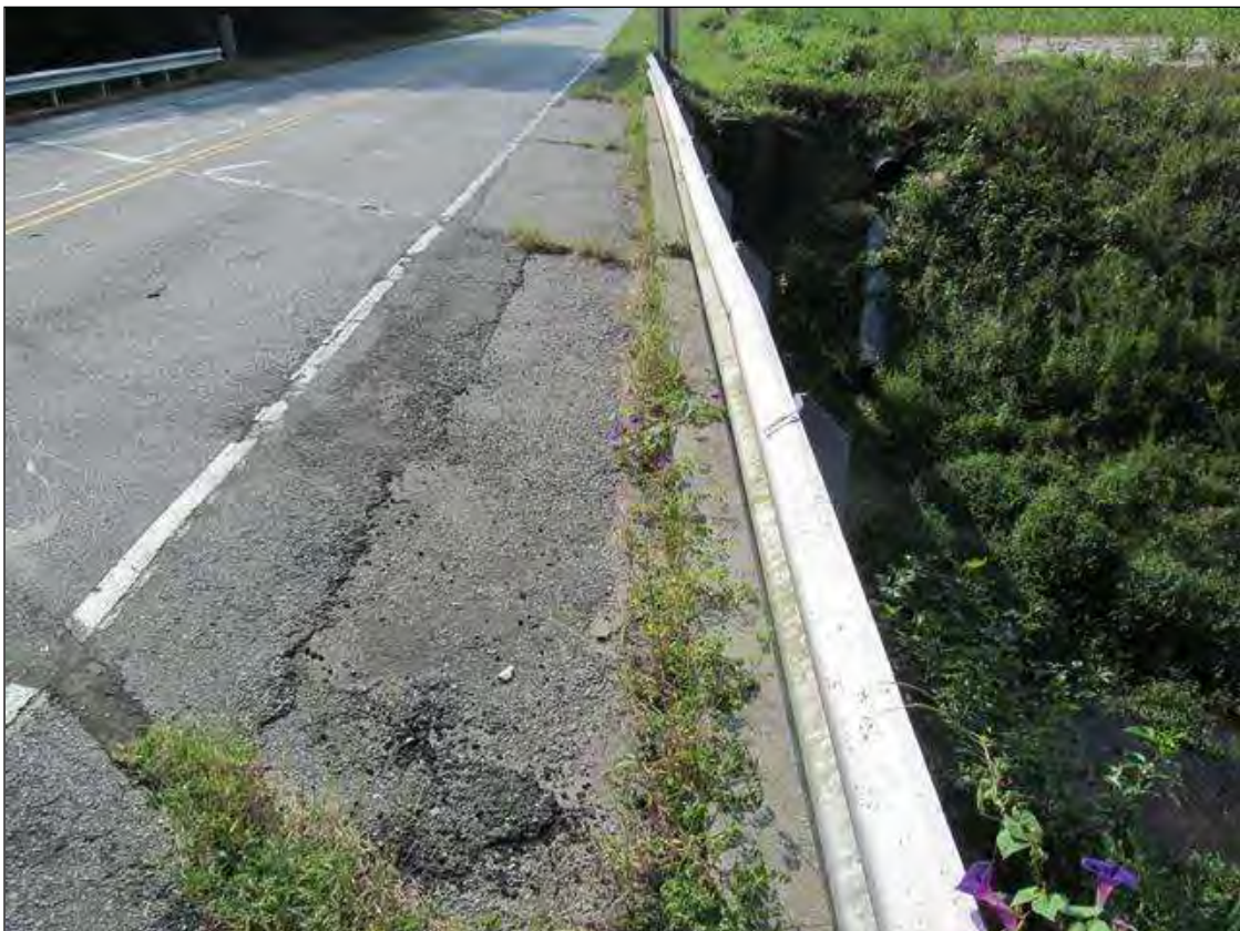
HEAVY VEGETATION ALONG RT CURB WITH BLOCKED DRAINS. SIMILAR ALONG LT SIDE.
