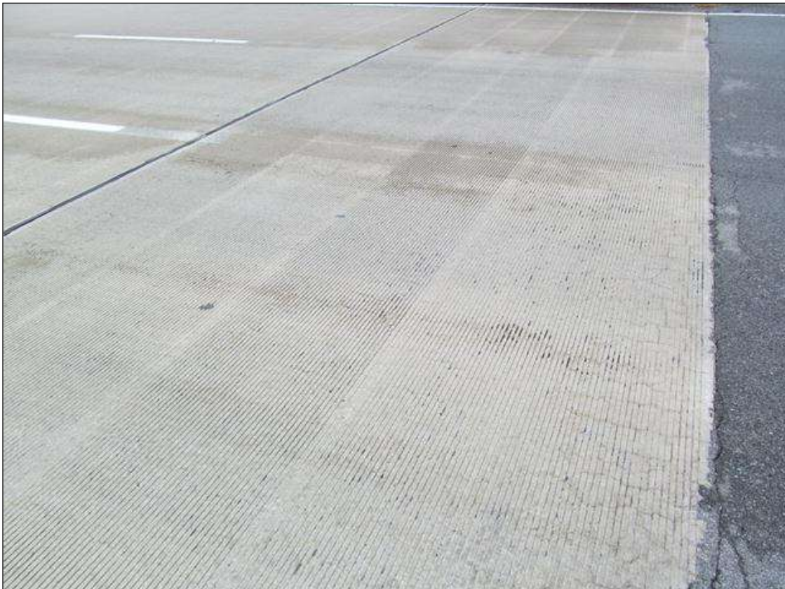
WEST APPROACH SLAB HAS CRACKS. THE EAST SLAB IS SIMILAR.
