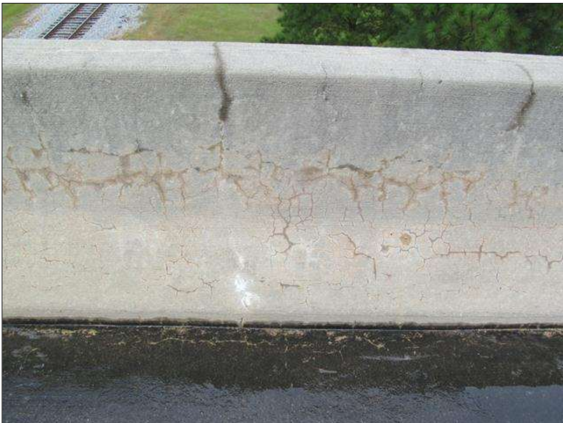
LEFT RAIL WITH CRACKS & SOME WITH EFFLORESCENCE. SIMILAR @ THE RIGHT RAIL.
