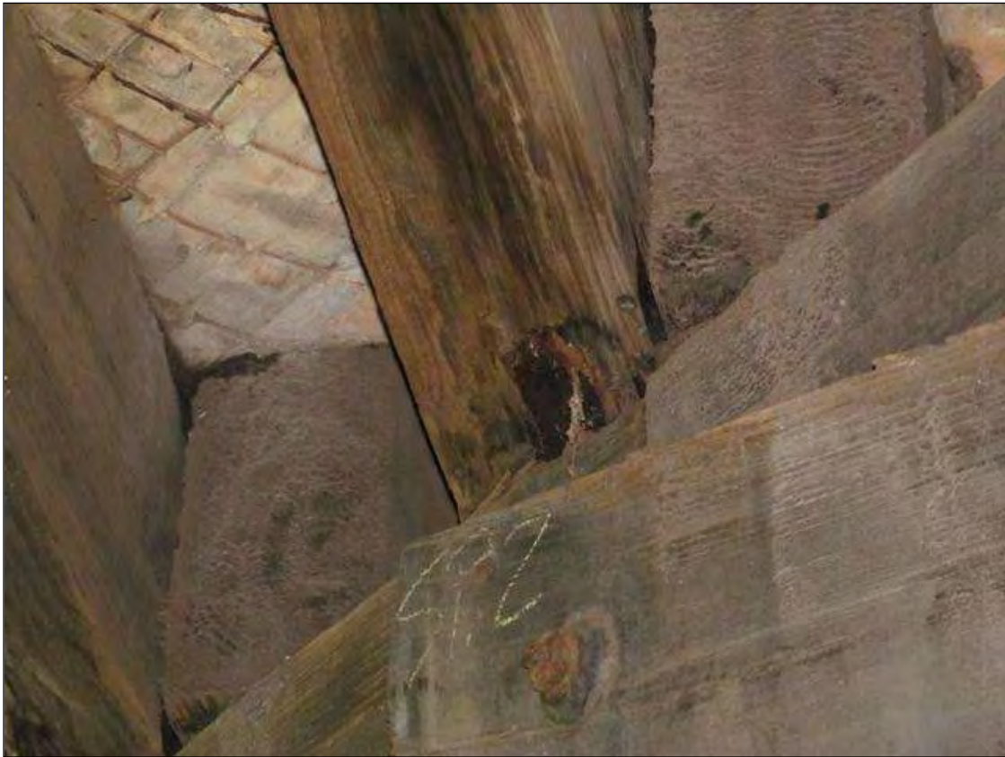
J-16 IN SPAN 2 DECAYED AT BEARING OVER BT 1
