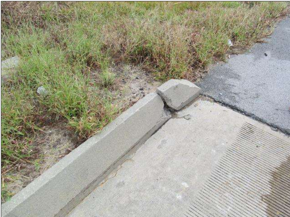
NE APPROACH CURB IS CRACKED AT END PORTION.
