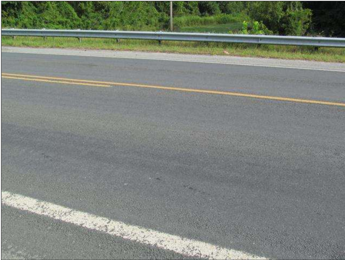
CRACKS & RUTTING IN THE WEARING SURFACE.
