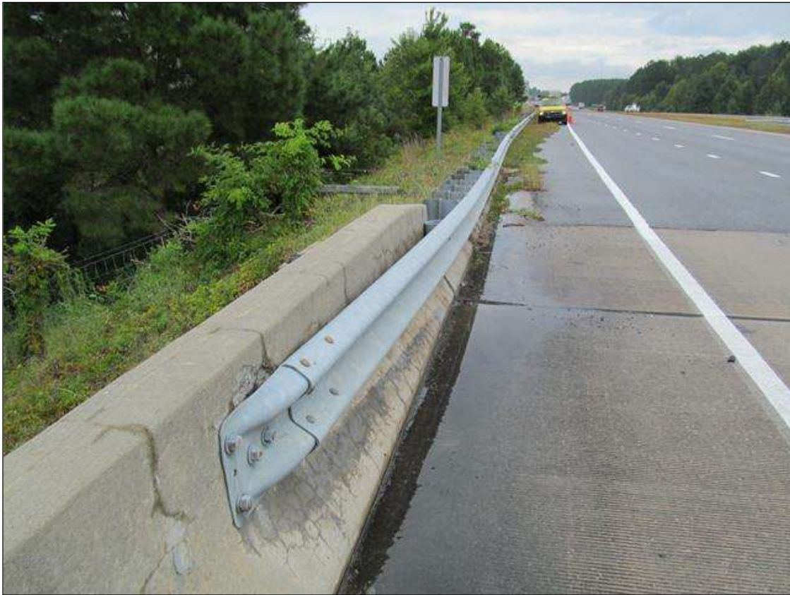
GUARDRAIL CONNECTION @ THE NE CORNER. SIMILAR @ THE SE CORNER.
