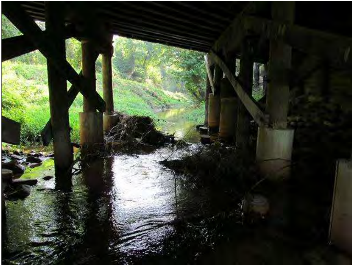
DRIFT IN SPAN 2
