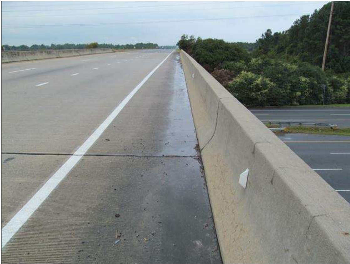
DEBRIS & PONDING ALONG THE LEFT RAIL. SIMILAR DEBRIS ALONG THE RIGHT RAIL.
