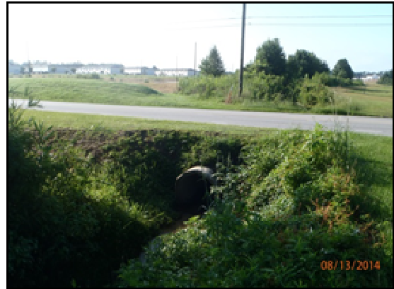
Picture 5-4: Perched culvert on north side of Thomas Langston Road
