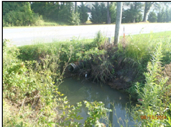
Picture 5-5: Exposed pipe on south side of Thomas Langston Road
