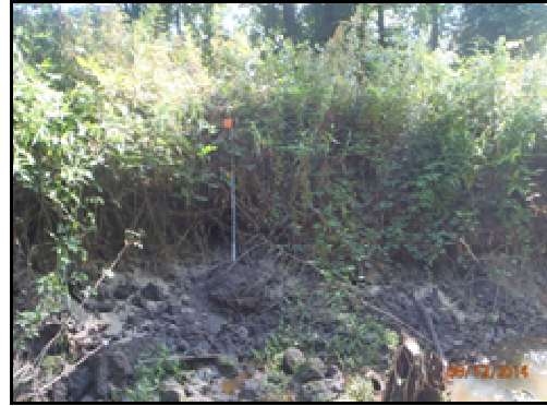
Picture 5-3: Erosion downstream of Thomas Langston Road
