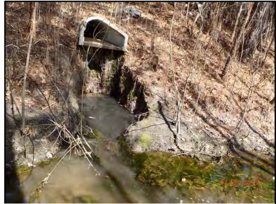
Picture 5-8. Exposed outfall on right bank
