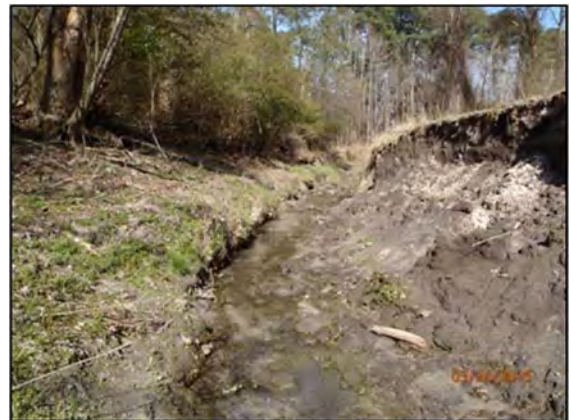
Picture 5-2. View from culvert at Live Oak Lane looking towards Fork Swamp
