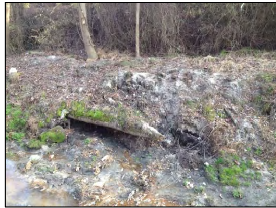
Picture 5-11. Failing log structures along right bank
