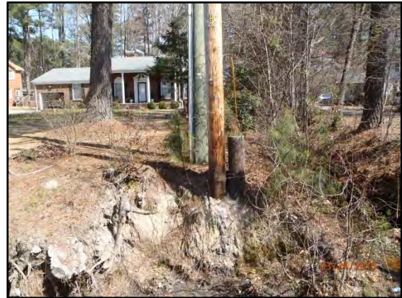
Picture 5-12. Eroding outfall and exposed telephone pole
