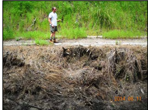
Picture 5-9. Eroding left bank between armored sections
