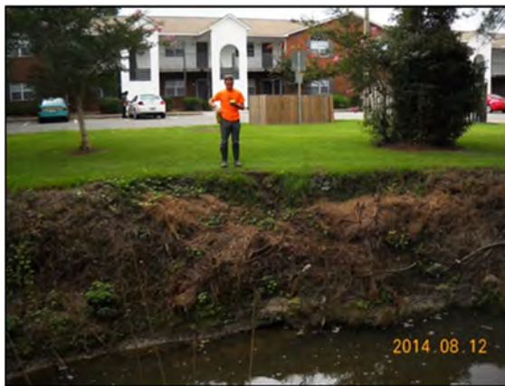
Picture 5-7. Erosion East of Tower Place
