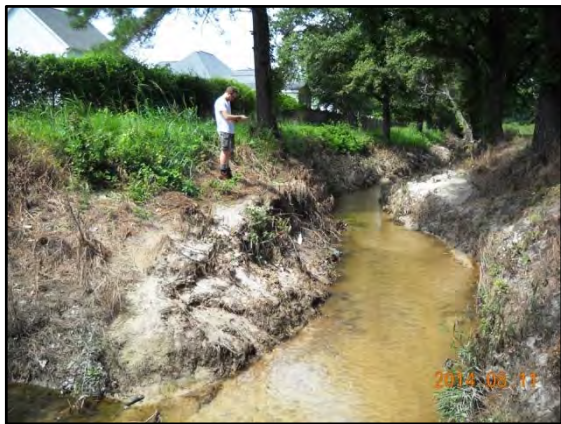
Picture 5-6. Erosion and lack of riparian buffer at Ashcroft outfall
