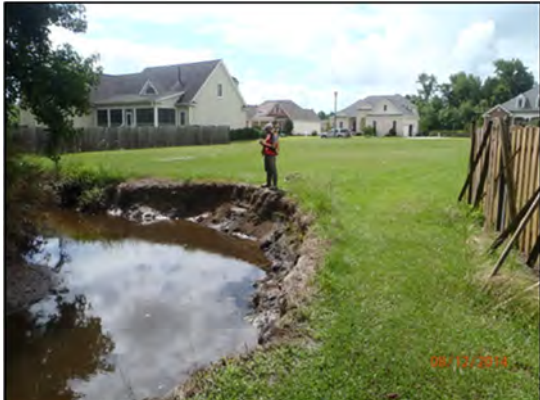
Picture 5-3. Eroding bank at 1205 Trafalgar Drive
