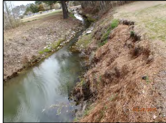
Picture 5-6. Erosion East of Tower Place
