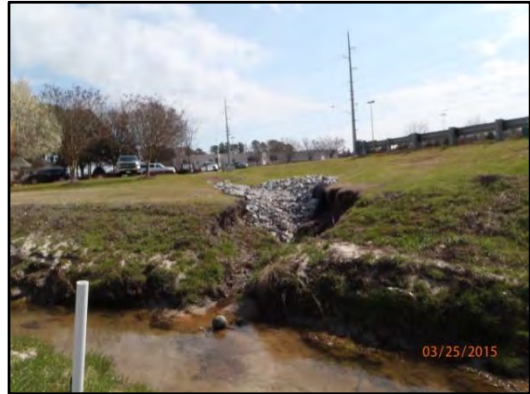
Picture 5-5. Highly eroded ditch at East Fire Tower Road
