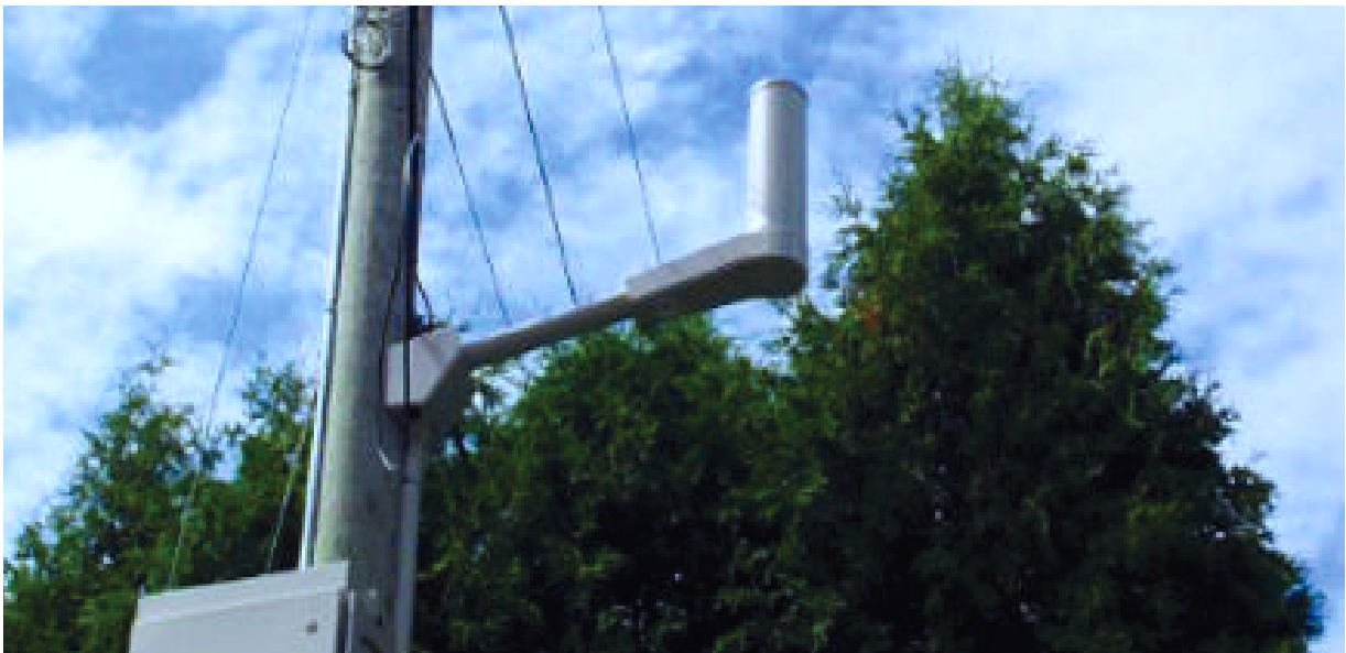
DAS and small cell antennas
