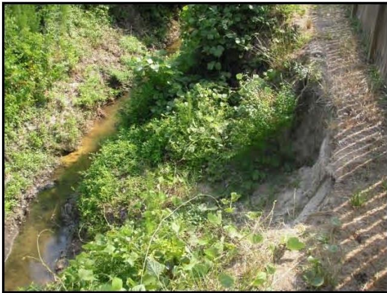
Picture 5-2. Severe bank erosion along landscaping fence
