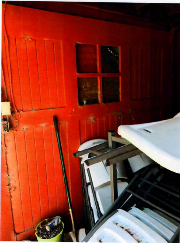
View of only remaining door, currently fixed in place along south wall.
