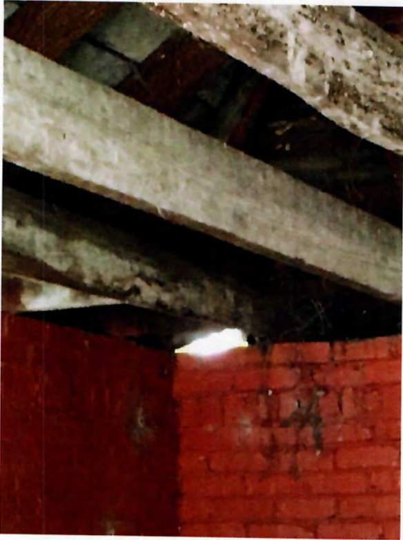
Interior view of south-west corner showing roof and rafter deterioration.
