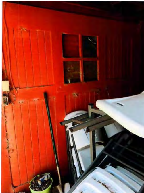
803 E Fifth Street – Remaining door used as an example
