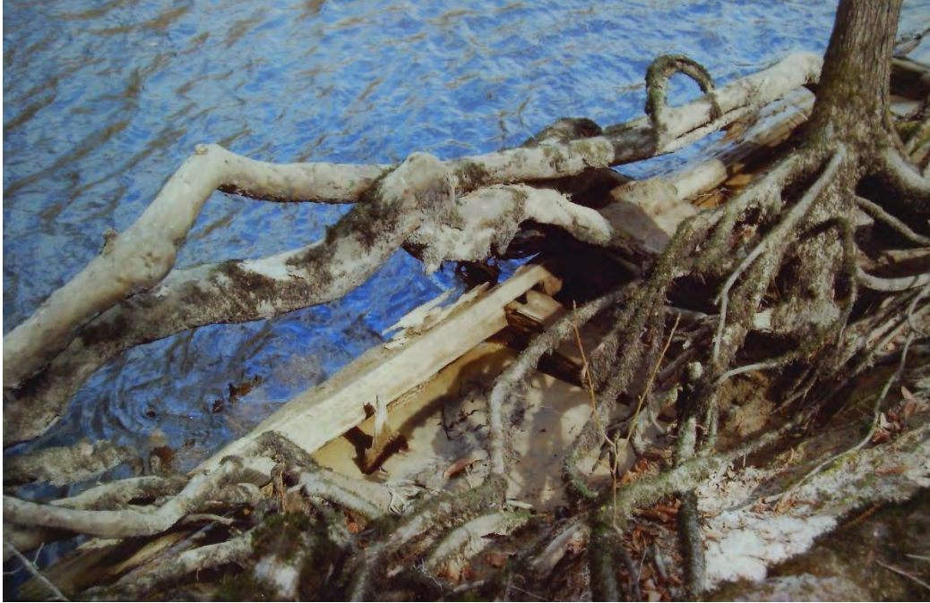
View of Overgrowth Covering Northern Edge. "Overgrowth_2" V. Bellis. 2017.
