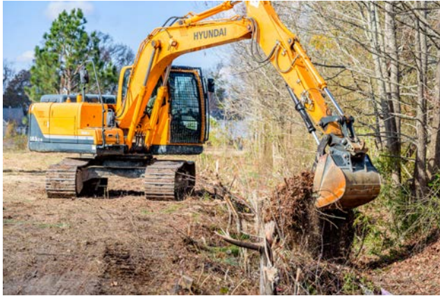
City stormwater crews removing stumps and clearing out debris from the ditch bottom.
