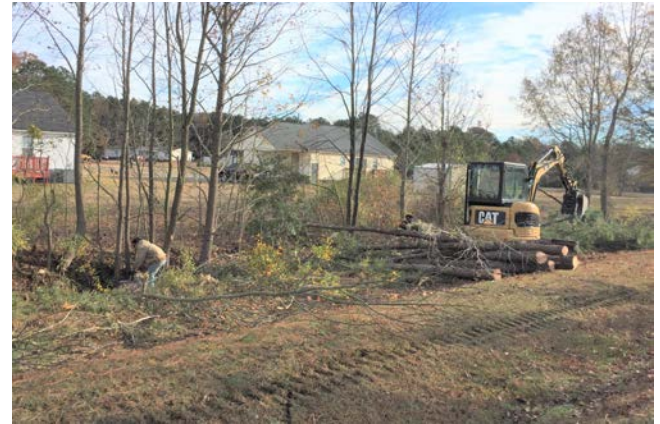
Contractor removing trees from the ditch line with a mini excavator and chainsaws.
