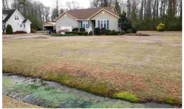
No guttering on structure; standing water in ditch
