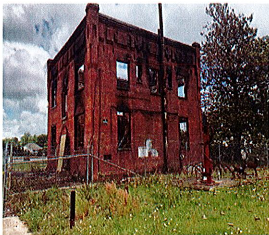
Figure 1 – Exterior View of Damaged Structure
