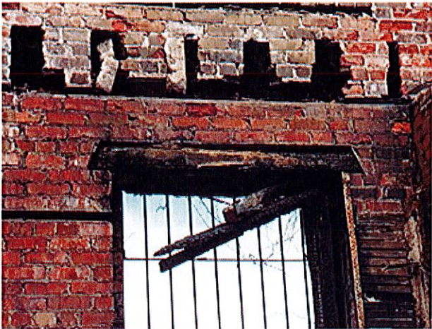
Figure 3 – Damaged Wood Lintel and Brick Spalling
