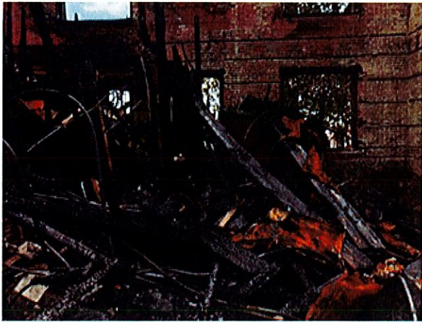
Figure 2 – Debris Covered Interior
