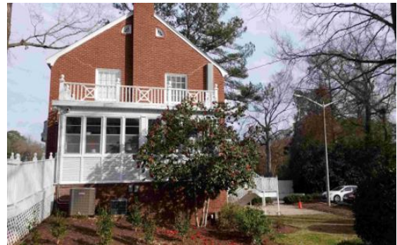
HVAC not elevated
