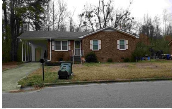
Guttering drains onto driveway
