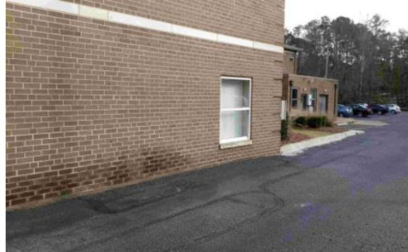
Visible water mark on side of apartment building
