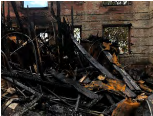
Figure 2 – Debris Covered Interior
