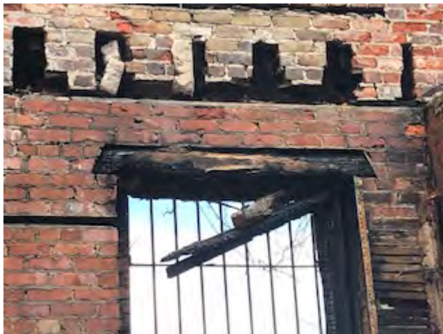
Figure 3 – Damaged Wood Lintel and Brick Spalling
