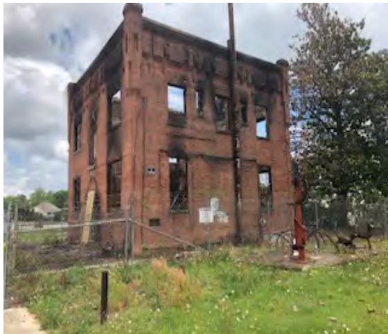
Figure 1 – Exterior View of Damaged Structure
