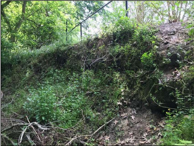
Section of erosion.
