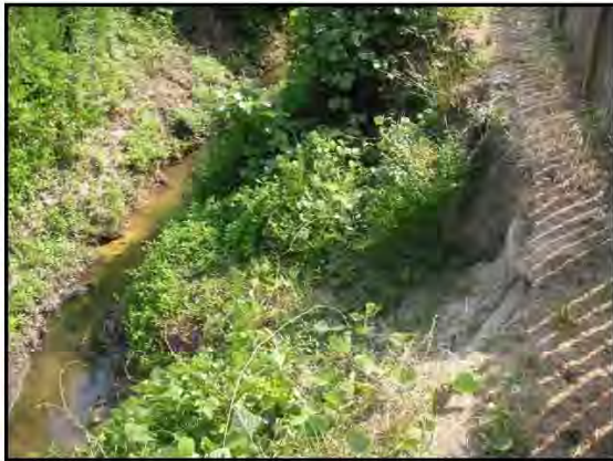
Picture 5-2. Severe bank erosion along landscaping fence
