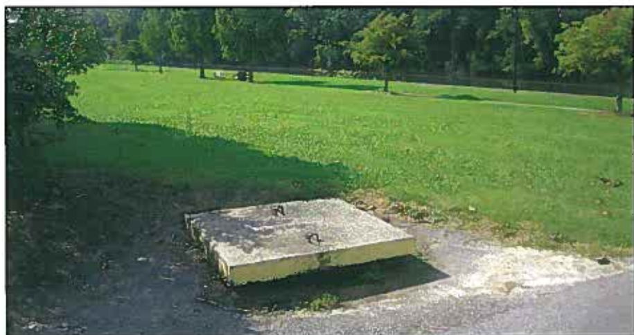
Storm drainage system; no BMP's
