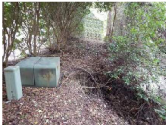
Picture 5-12: Electric Transformers at Top of Bank
