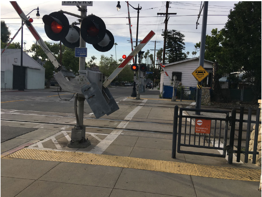
A pedestrian crossing in Los Angeles on the Metro Gold Line includes automatic pedestrian gates and emergency exit swing gates. Where geometrically feasible, they are attached to the same assembly as the roadway gates for cost savings.
