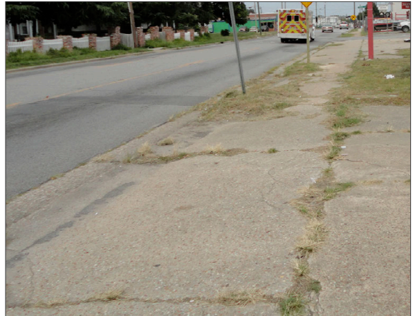
Some sidewalk are cracked, overgrown and/or are no longer level. Above: Sidewalk on Dickinson Avenue.
