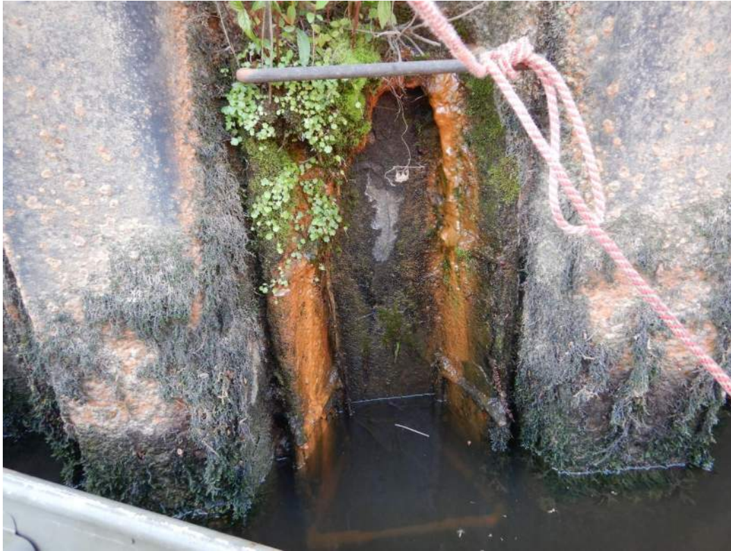
PHOTOGRAPH 2.11: MISSING BOTTOM RUNGS OF AN ACCESS LADDER (STATION 11+65)
