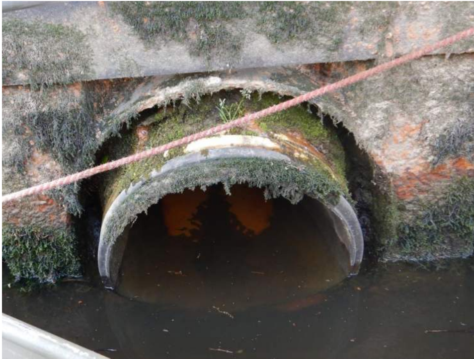
PHOTOGRAPH 2.8: CONDITION OF CMP OUTFALL AND STEEL PIPE SLEEVE (STATION 10+38)
