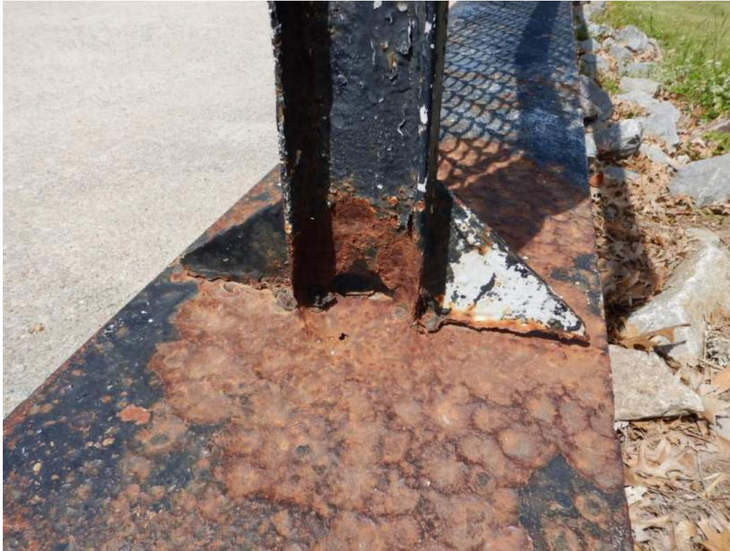
PHOTOGRAPH 2.4: CONDITION OF FIRST HANDRAIL POST (STATION 0+02)
