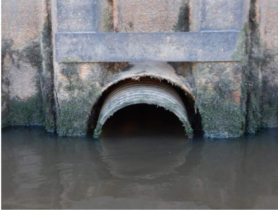
PHOTOGRAPH 2.9: CONDITION OF CMP OUTFALL AND STEEL PIPE SLEEVE (STATION 4+18)
