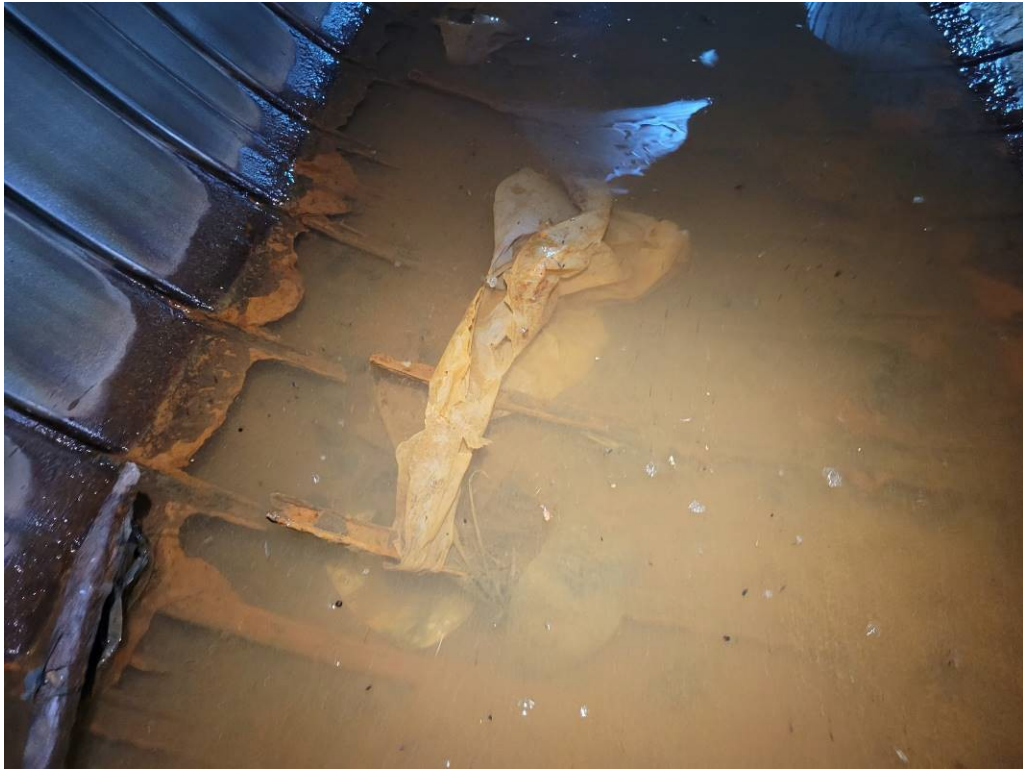
Photo 27 Sta 10+92 Severe corrosion with up to 6" of soil erosion
