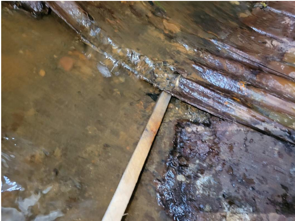
Photo 10 At MH base, erosion under pipe, sta 1+90
