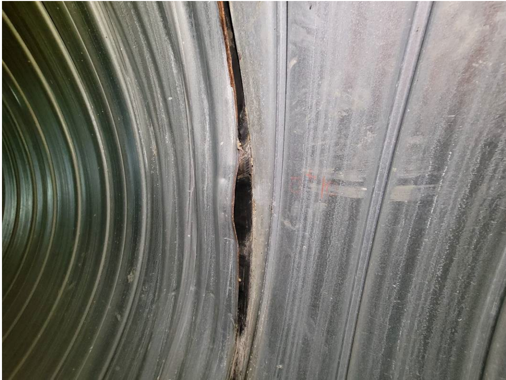
Photo 7 Damaged joint in corrugated steel pipe (CSP), sta 0+10
