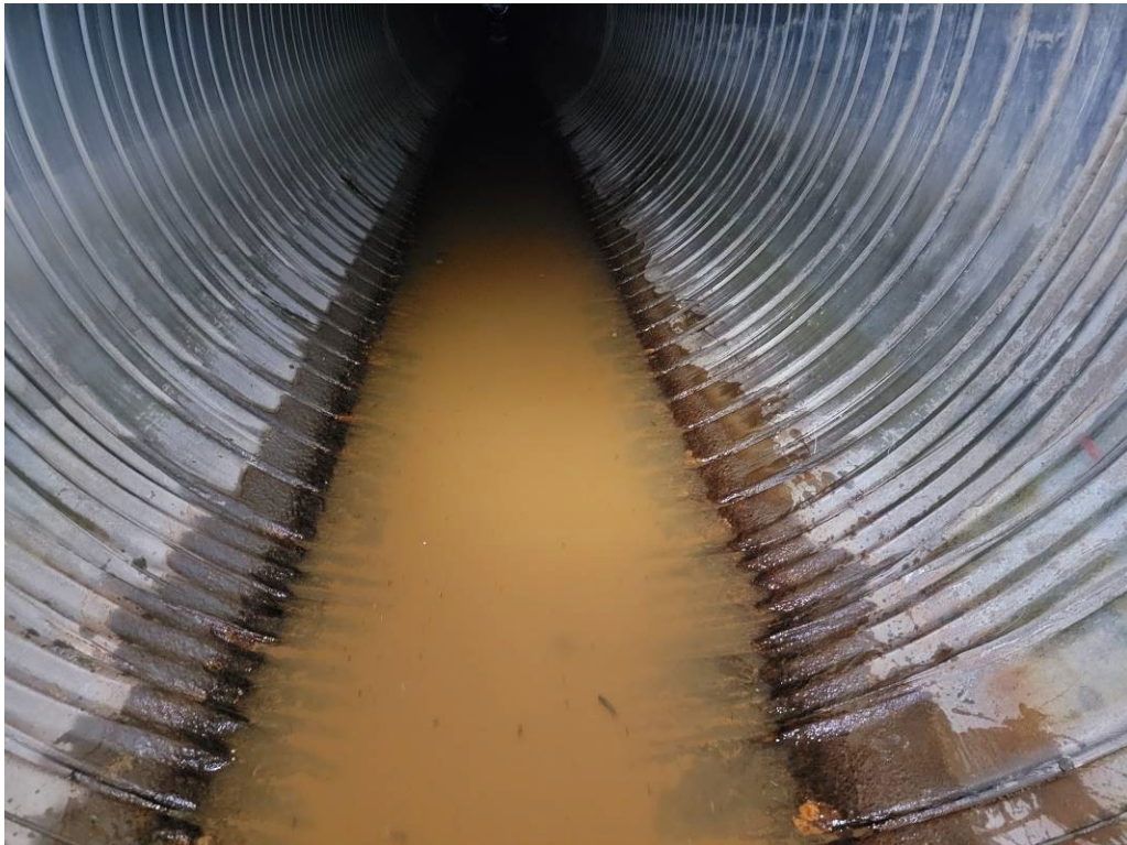
Photo 30 Sta 14+00 Moderate corrosion
