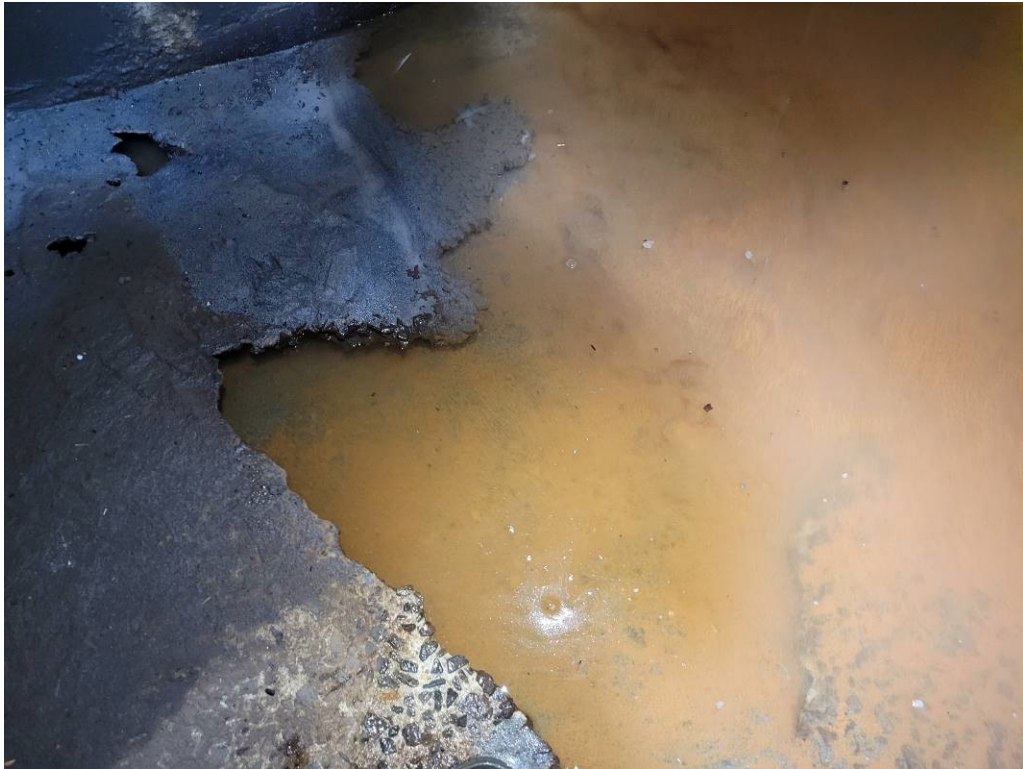
Photo 29 Sta 13+56 Manhole basin; severe erosion of concrete floor
