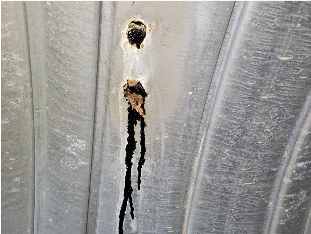
Photo 11 Sta 1+91, apparent repair with sealant showing, approximately 11 o'clock
