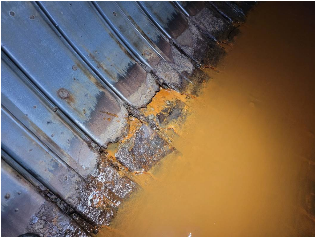
Photo 24 Station 9+45 Severe corrosion, breached pipe
