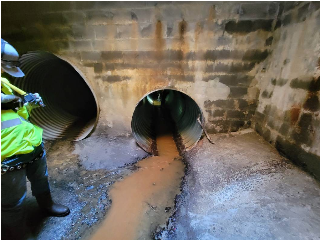
Photo 34 Sta 15+54 Manhole with second 84" entrance, 54" exit (presumed to be at or near railroad)
