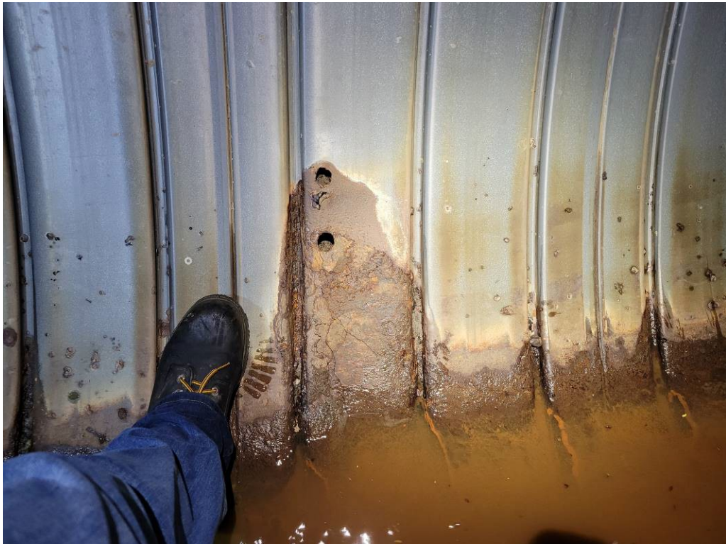
Photo 16 Sta 4+94 Severe corrosion breaching the pipe with visual evidence of soil erosion
