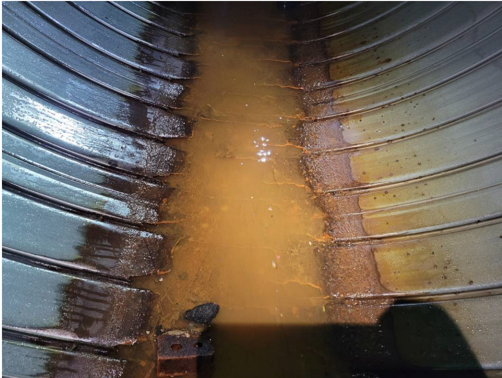
Photo 13 Sta 3+27, sever corrosion at flow line. Pipe breached at most flutes
