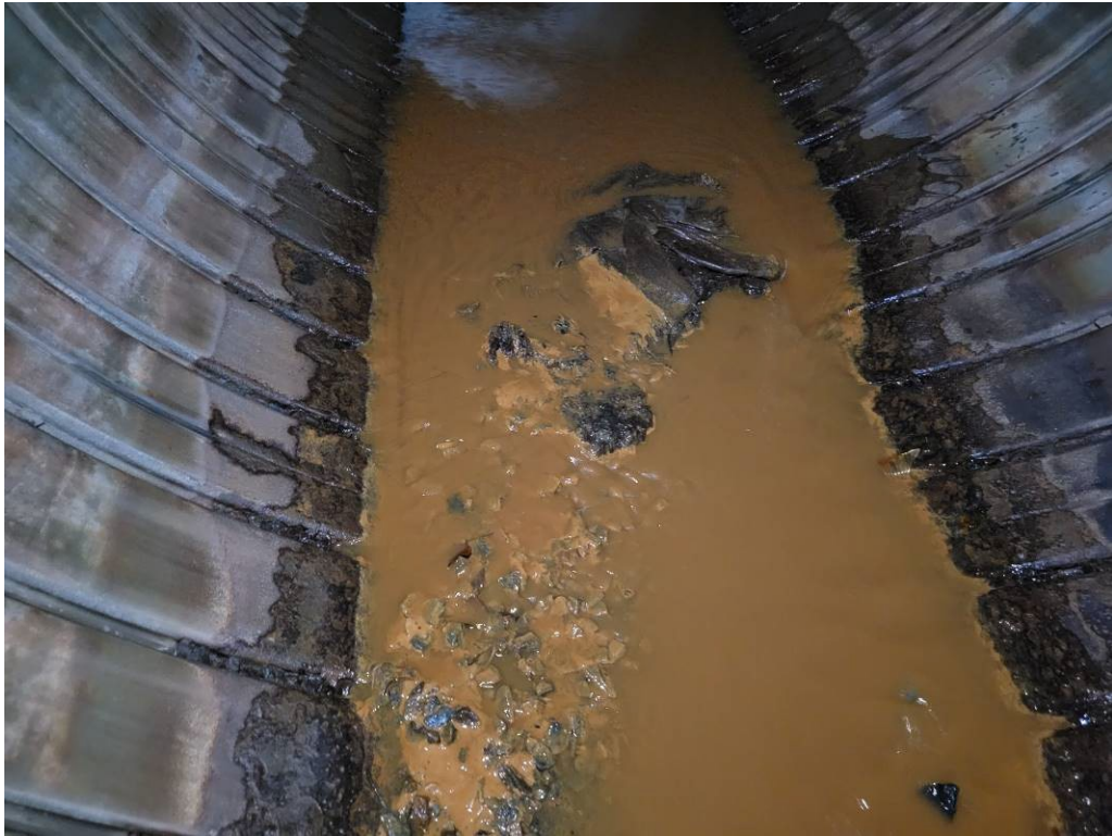
Photo 33 Sta 14+62 Significant sediment and debris
