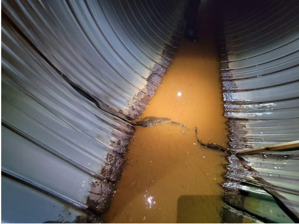
Photo 19 Sta 6+82, severe corrosion with gasket displaced
