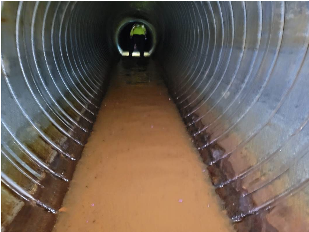
Photo 38 Sta 18+00 Minor corrosion. Smell of diesel
