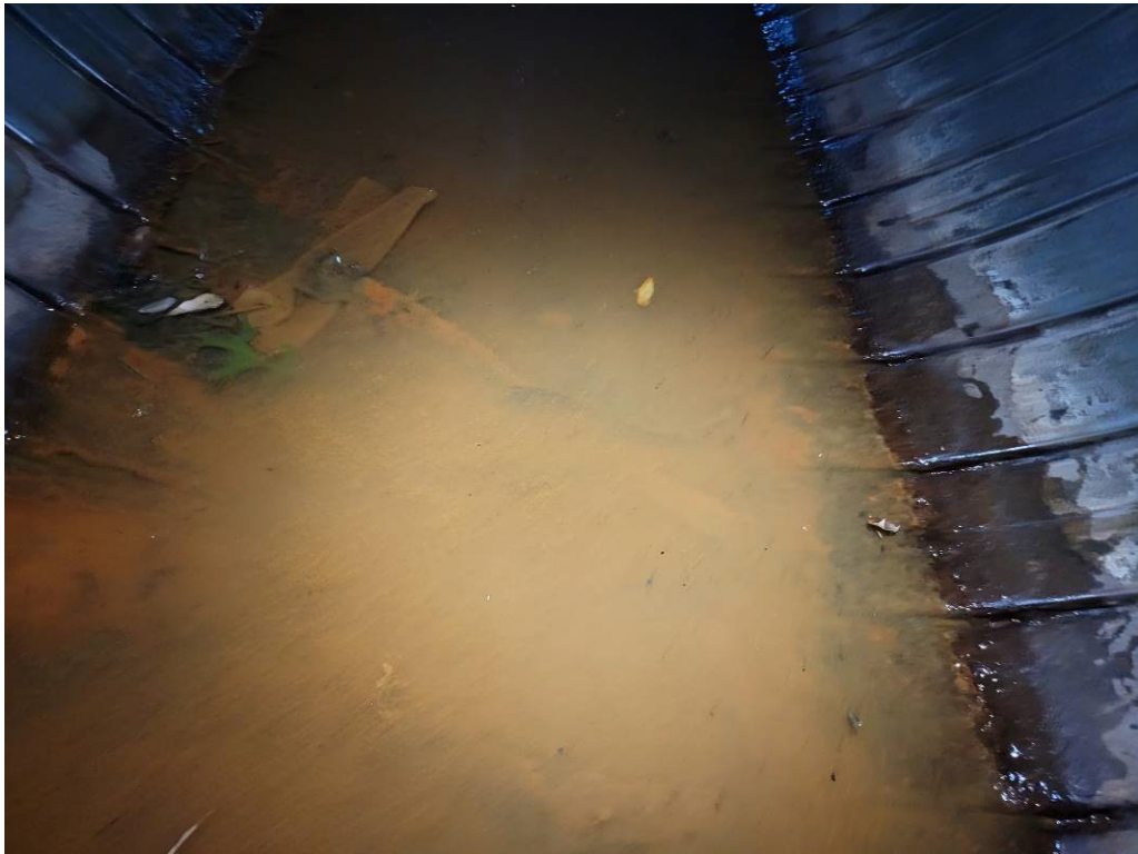
Photo 26 Sta 10+80 Severe corrosion with CSP flutes displaced
