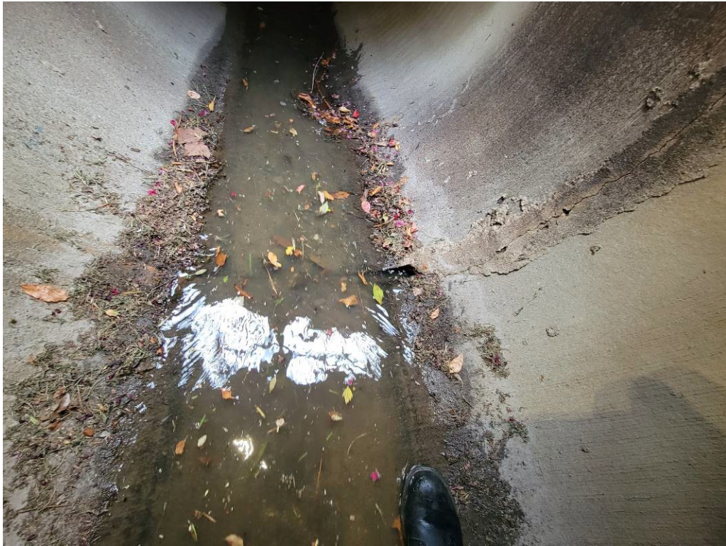
Photo 3 Water level in RCP. Note deteriorating joint
