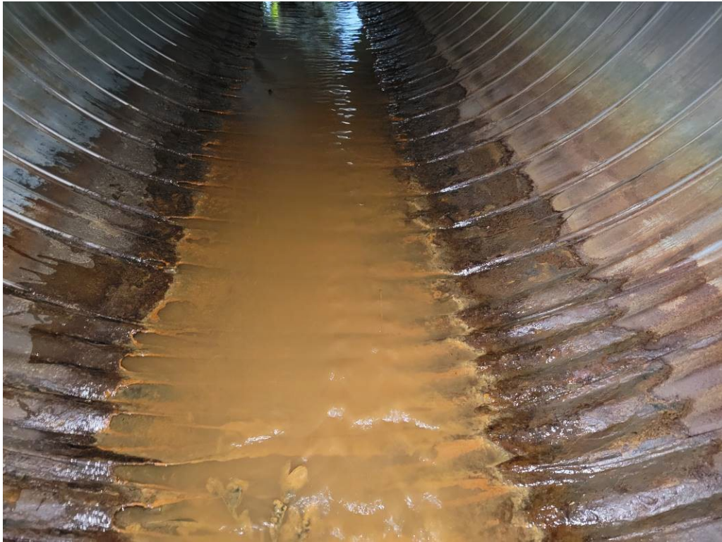
Photo 31 Sta 14+10 Severe corrosion with penetrations
