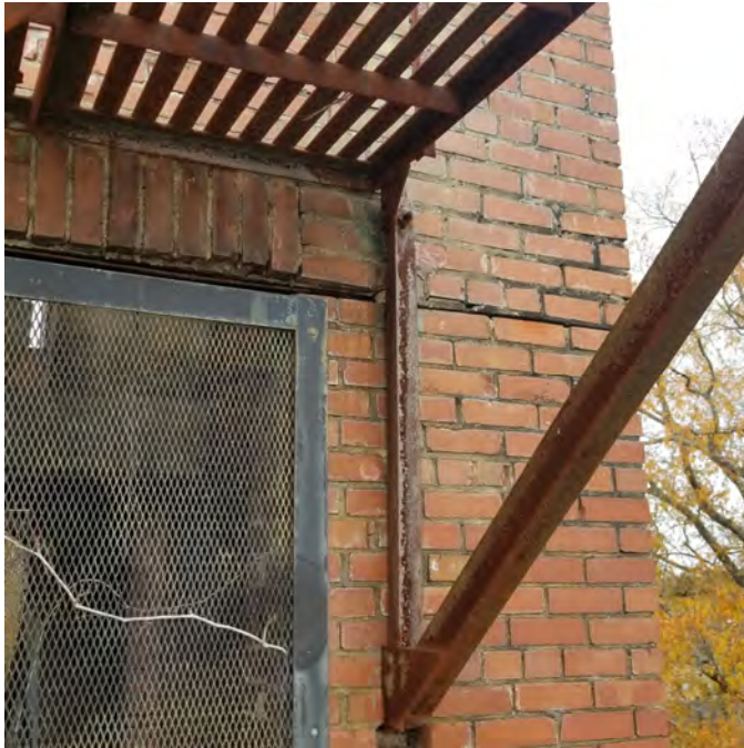
PHOTOGRAPH NO. 14: LINTEL CORROSION
