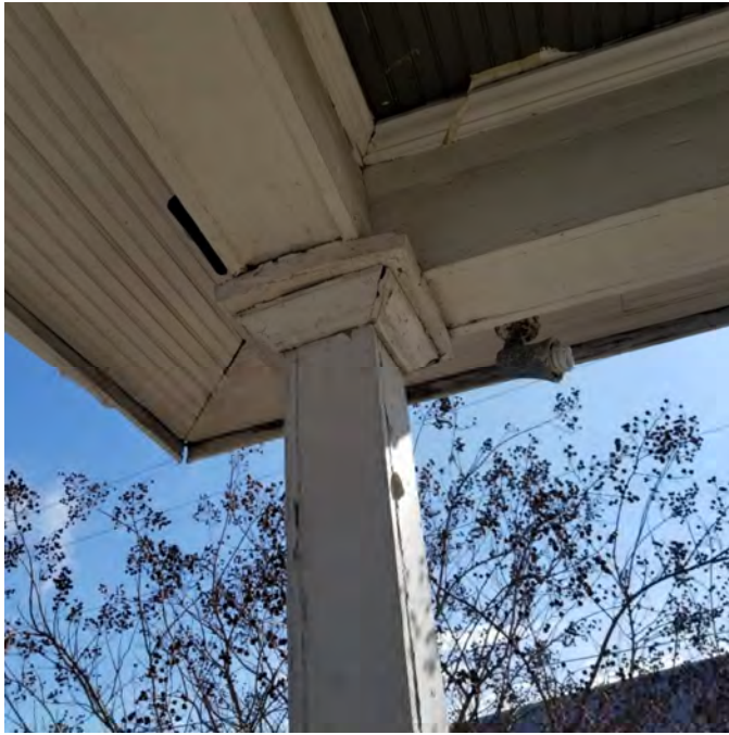
PHOTOGRAPH NO. 37: DETERIORATED ENTRY COLUMN AT TOP
