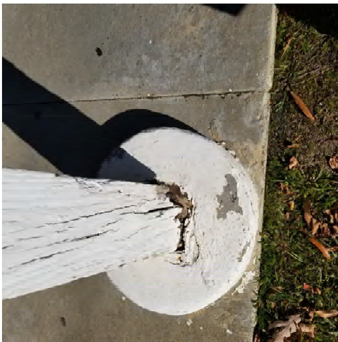
PHOTOGRAPH NO. 36: DETERIORATED ENTRY COLUMN AT BASE
