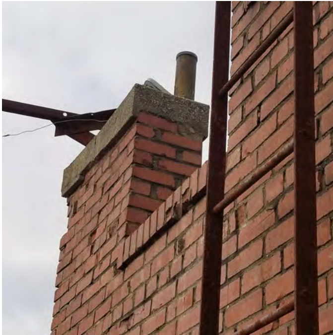
PHOTOGRAPH NO. 18: DAMAGED PARAPET BRICK
