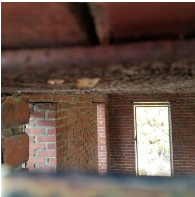
PHOTOGRAPH NO. 21: INTERIOR VIEW SHOWING DAMAGED BRICK
