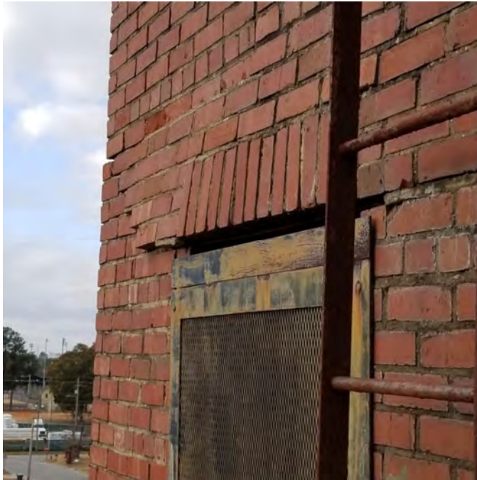
PHOTOGRAPH NO. 16: BRICK SHIFTED/UNSTABLE
