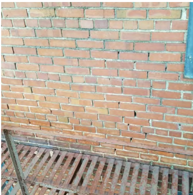
PHOTOGRAPH NO. 15: MORTAR DETERIORATION
