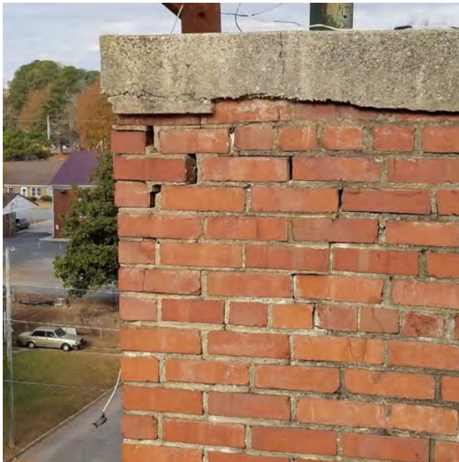
PHOTOGRAPH NO. 19: LOOSE BRICK AT PARAPET
