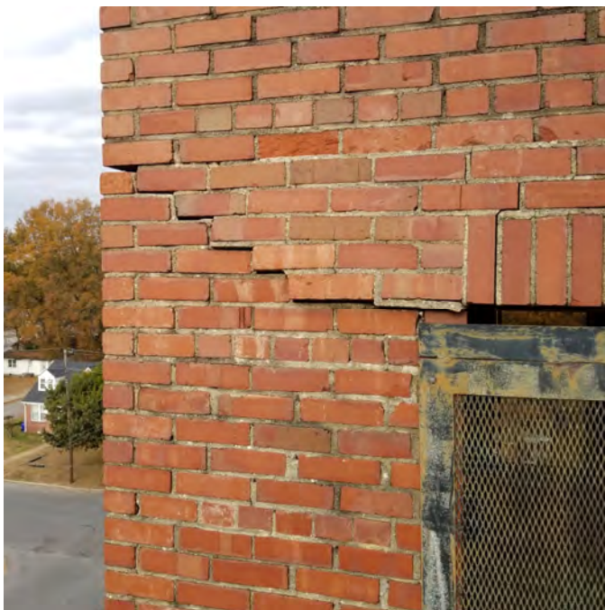
PHOTOGRAPH NO. 17: BROICK SHIFTED/UNSTABLE
