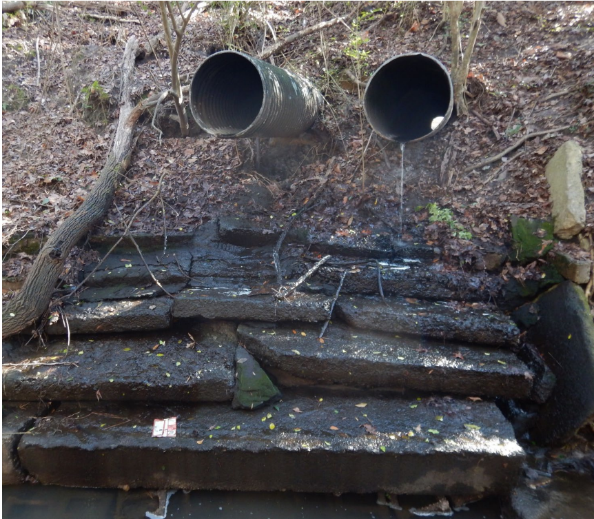
Aging stormwater outfall pipes
