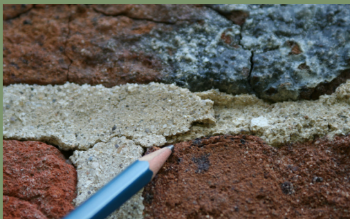
A close-up photograph of defective repointing indicating the edge of the newer mortar and the original mortar exposed to the right.
