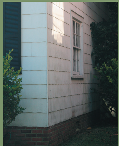
Promoted for their fire resistance, asbestos shingles were one of the early kinds of synthetic siding. Several houses in the CVHD retain their original asbestos shingles.
