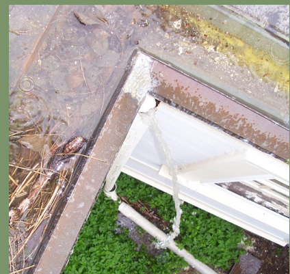
During a rainstorm, a gutter's failed connections show themselves. Take the opportunity to inspect roofs and gutters when its raining.
