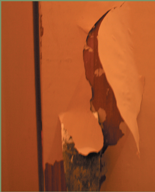
After heating with an infrared paint remover, paint is easily scraped away. This method is especially efficient for removing paint from previously varnished surfaces like doors.
