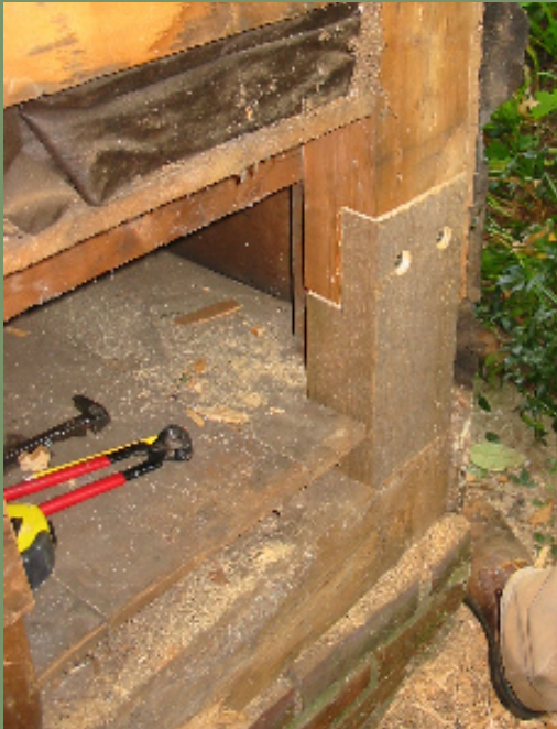
A large scale Dutchman repair secured with a lap joint and bolts. Smaller Dutchman repairs are typically held by their tight fit and glue, with no fasteners.
