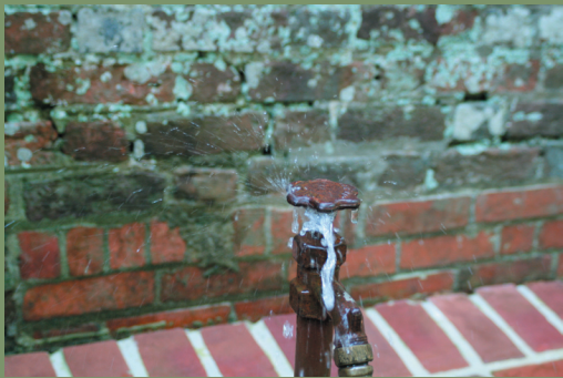
To avoid having to repoint masonry, keep it dry! In the above photograph, a leaky faucet has been routinely spraying the historic masonry wall behind it every time the sprinkler system goes off. As a result, lichen is thriving on the wall and the bricks and mortar deteriorated. A bad repair was then made with completely incompatible modern bricks and mortar, but the primary cause of the problem remains unaddressed.
