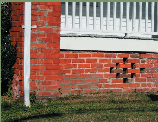
Three examples of foundation ventilation found in the College View Historic District. Two styles of pierced brickwork and a modern louvered ventilator. Foundation ventilation is an important part of limiting moisture collection beneath a house.
