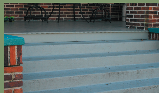
The deteriorated portion of the above porch floor was properly repaired and repainted as part of a COA project.
