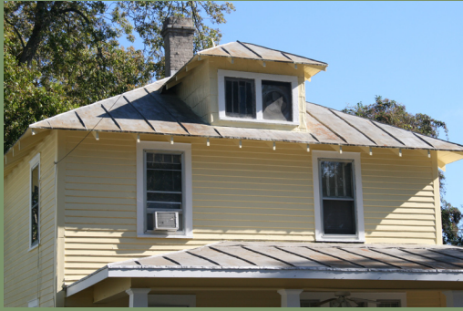
An example of a standing seam roof in the College View Historic District. This home also retains pressed tin shingles on its dormer.
