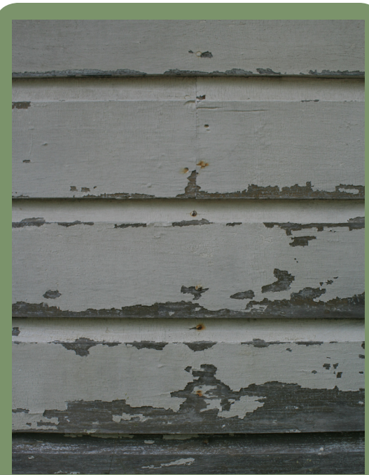
The rust of nail heads will emerge through a new paint job if not pretreated. Touch nail heads with a rust inhibiting priming prior to priming the rest of the wall or element. Avoiding the defacing rust that can appear after the paint job is done is a big payoff for this simple step.
