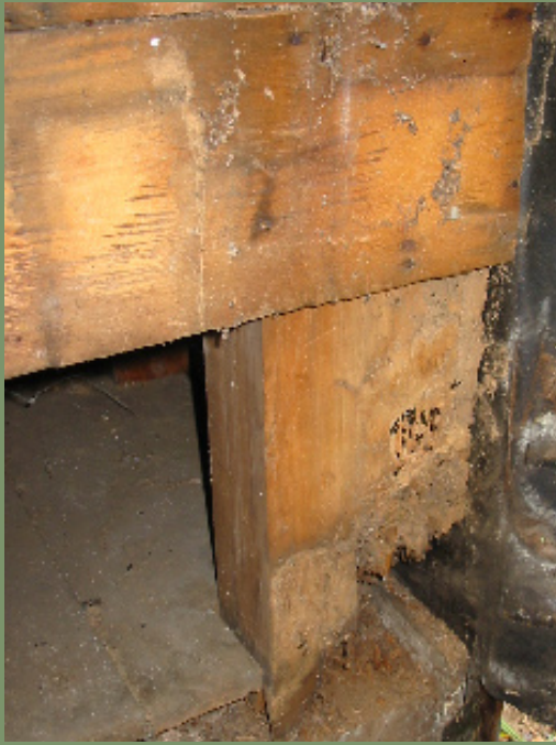
The bottom end of a corner post mostly lost to rot.
