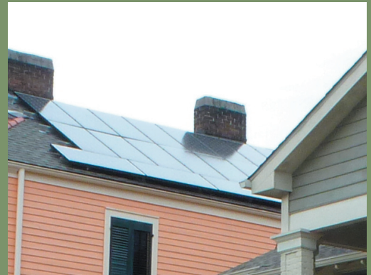
The character defining front roof slope of the above house retains its original appearance, while solar panels are appropriately installed on a secondary slope. Photographs courtesy Heather Knight.
