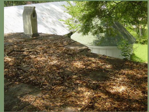
A flat roof covered in organic debris from an adjacent tree. Flat roofs are especially prone to the accumulation of organic material which holds moisture against the roofing and leads to its degradation. A push broom should be used to clear roofs of plant debris. Trees should also be pruned to keep branches off of direct contact with the roof or other parts of the house.
