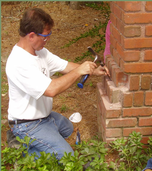
A Preservation Trades student of Edgecombe Community College cleans a joint in preparation for repointing. Note that eye protection should always be worn when doing this work. Photograph courtesy Monika Fleming.
