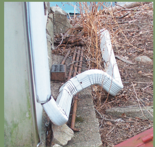
Good gutter design and maintenance is essential to avoiding foundation problems. Here, a poor attempt to repair a gutter leaves water funneling directly against the foundation.
