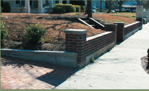
This brick retaining was newly constructed as part of a COA project. Through its proportions, design, and materials it blends in appropriately with the existing streetscape.
