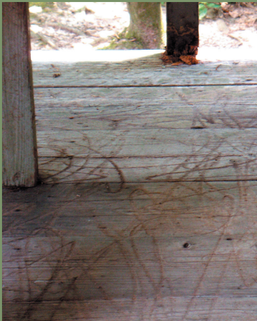
Close-up of pressure washer damage.
