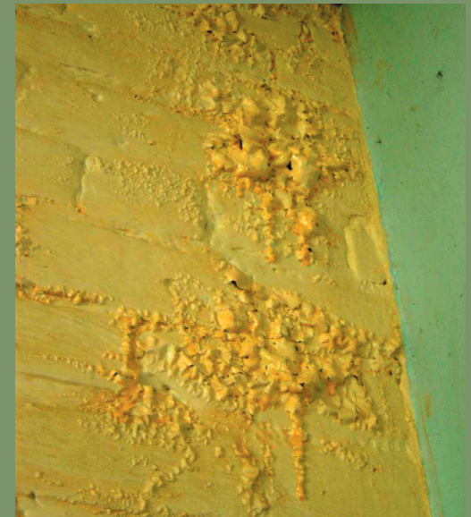
A peroxide-activated stripper at work on a tough old paint coating over brick. This variety of strippers is effective and user friendly. See masonry section.
