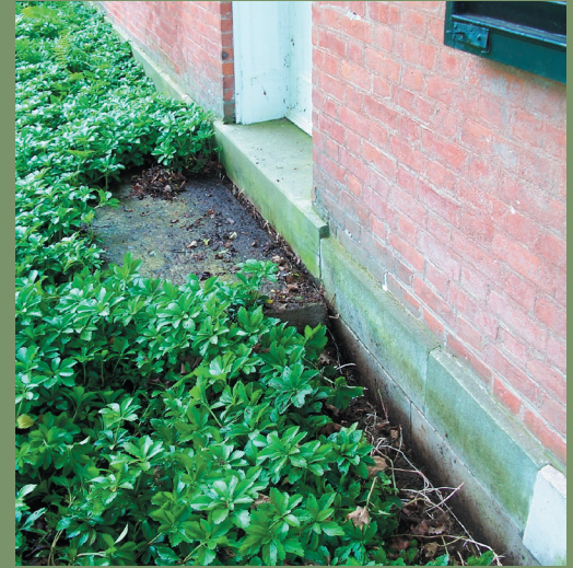
Vegetation should be kept off of foundations. At the above property, pachysandra was allowed to grow against the foundation, contributing to moisture issues. On the right, the vegetation has been cut back, revealing the line of biological growth that thrived on the granite in the moist environment.
