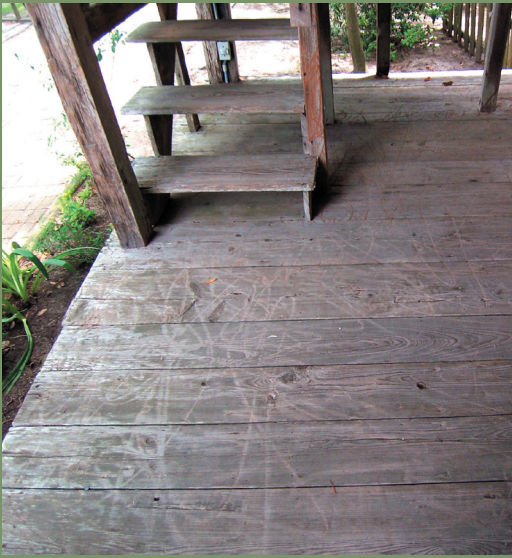
Pressure washer damage is evident on this wood porch floor.
