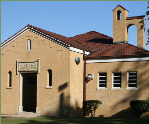
The red clay tile roof of the Third Street School is a defining feature of its Spanish Colonial Revival style.
