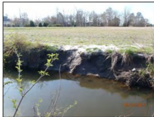
Figure 12. Erosion and lack of riparian buffer downstream of Corey Road
