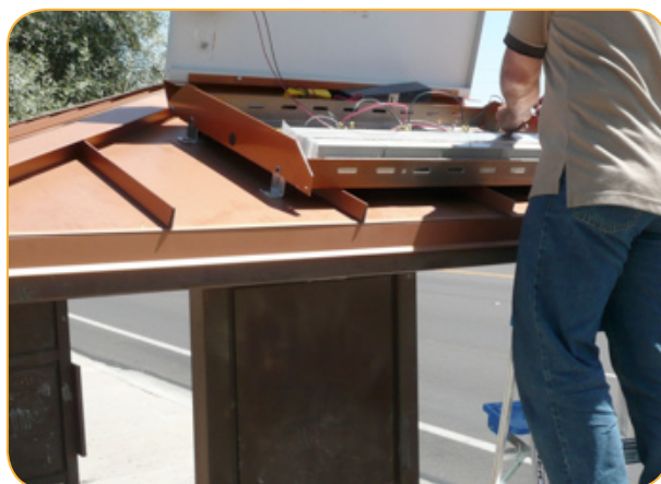
figure 4. Open roof mounted RMS
