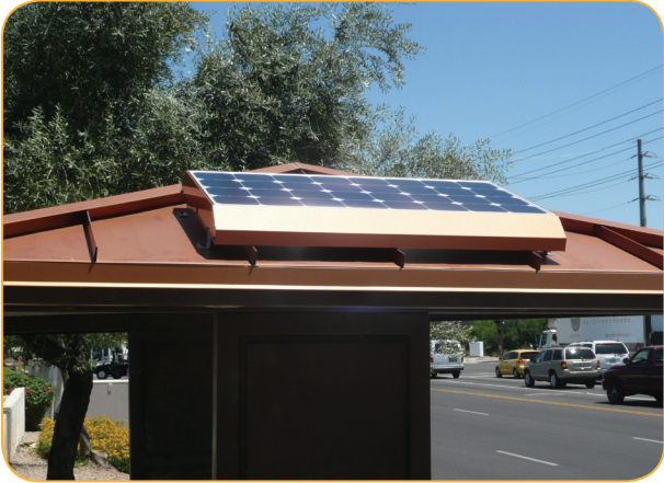
figure 2. Power module mounted on shelter
