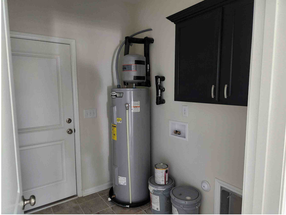
LAUNDRY ROOM / WATER HEATER
