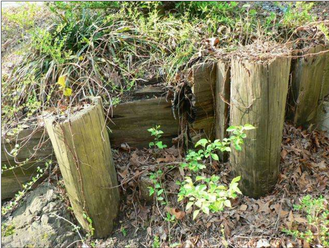
AREAS OF DECAY IN SOUTHEAST WINGWALL
