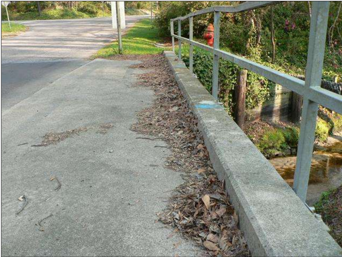
DEBRIS ACCUMULATION ALONG DOWNSTREAM CURB
