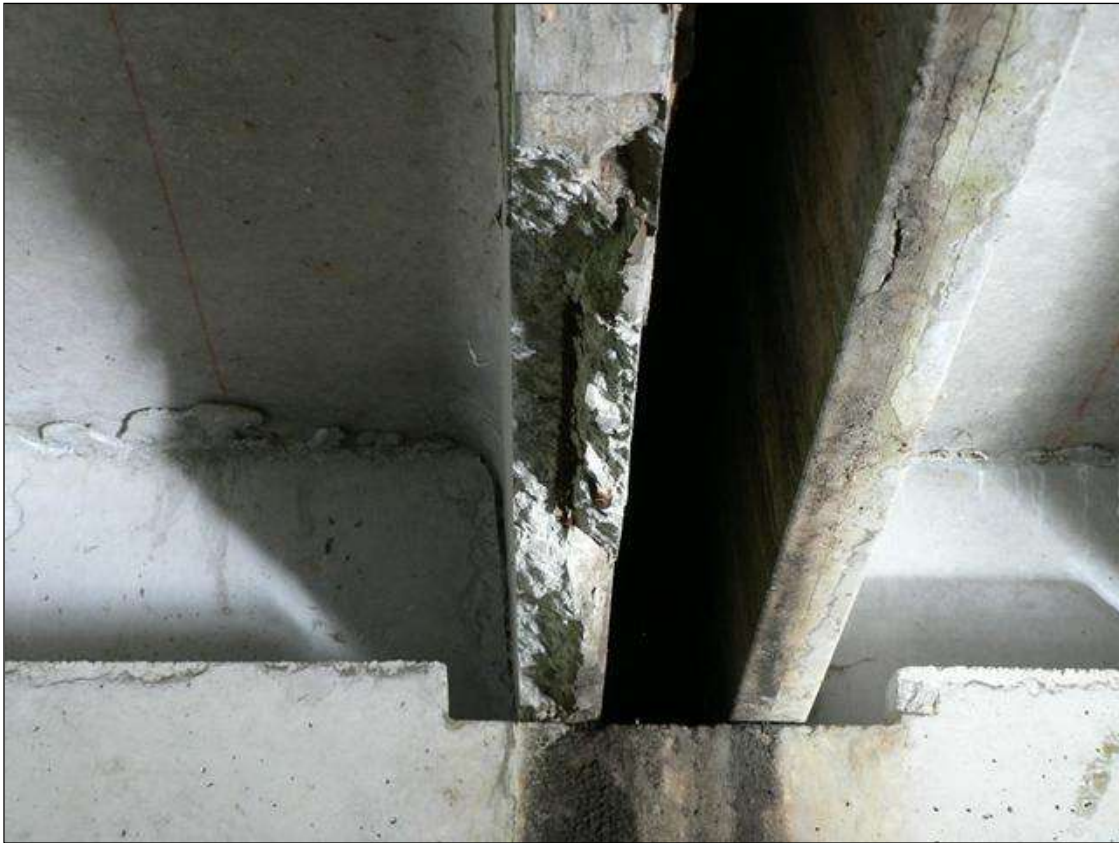
30" X 3" X 2" DEEP SPALL WITH EXPOSED STRAND IN LEG 2 OF CHANNEL 5 AT END BENT 2 (PRIORITY MAINTENANCE)
