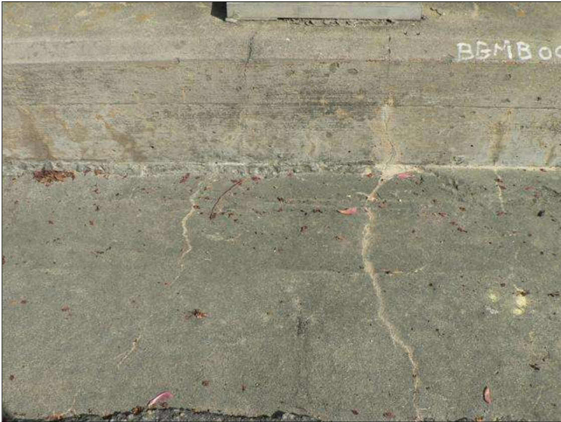
VERTICAL HAIRLINE CRACK WITH EFFLORESCENCE IN FACE OF DOWNSTREAM PARAPET EXTENDING INTO TRANSVERSE HAIRLINE CRACK IN TOP OF DECK AT RAIL POST 4
