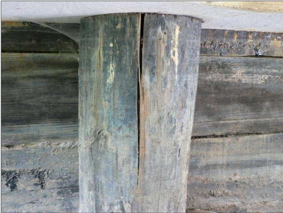
UP TO 1/4" SPLIT IN PILE 2 AT END BENT 2
