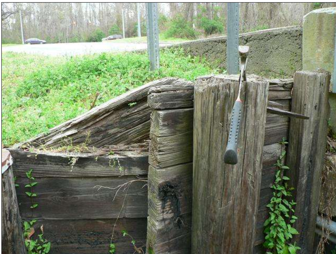
78" X 4" WIDE AREA OF DECAY IN NORTHWEST WINGWALL
