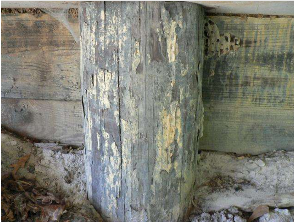
CHECKS AND SPLITS IN PILE 5 AT END BENT 1
