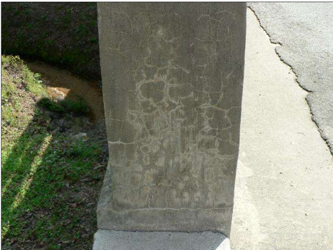
HAIRLINE MAP CRACKING WITH EFFLORESCENCE IN WEST FACE OF DOWNSTREAM END POST AT END BENT 1
