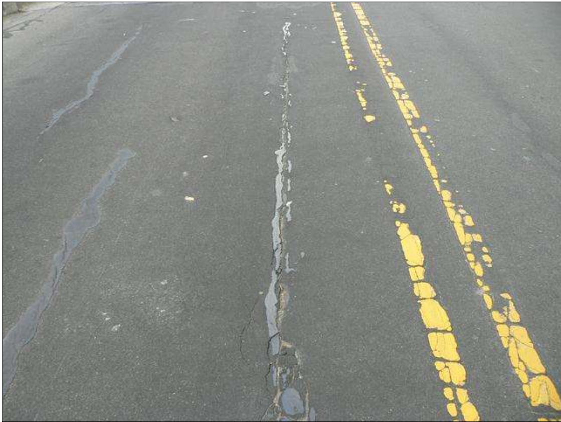
LONGITUDINAL REFLECTIVE CRACKS IN ASPHALT WEARING SURFACE IN SOUTHBOUND LANE
