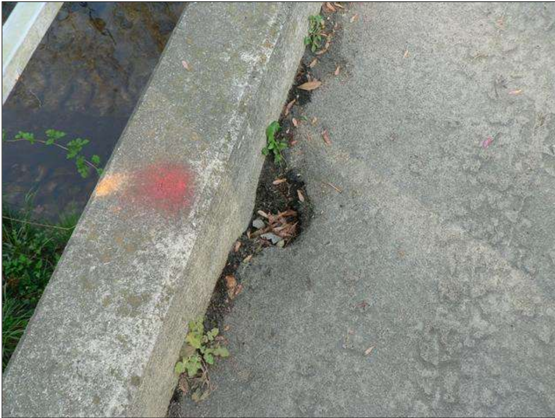
CLOGGED DECK DRAIN AT UPSTREAM CURB NEAR SOUTH END
