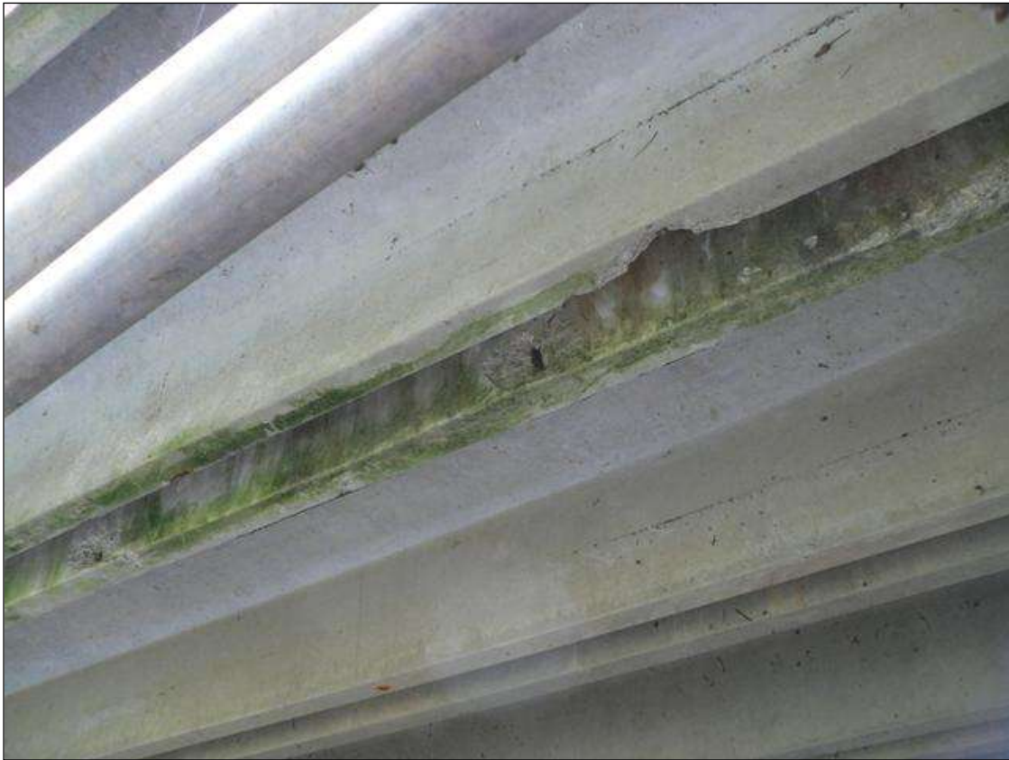
TWO 5" X 4" X 1/8" DEEP SPALLS WITH EXPOSED STIRRUP IN UPSTREAM FACE OF LEG 1 IN CHANNEL 2
