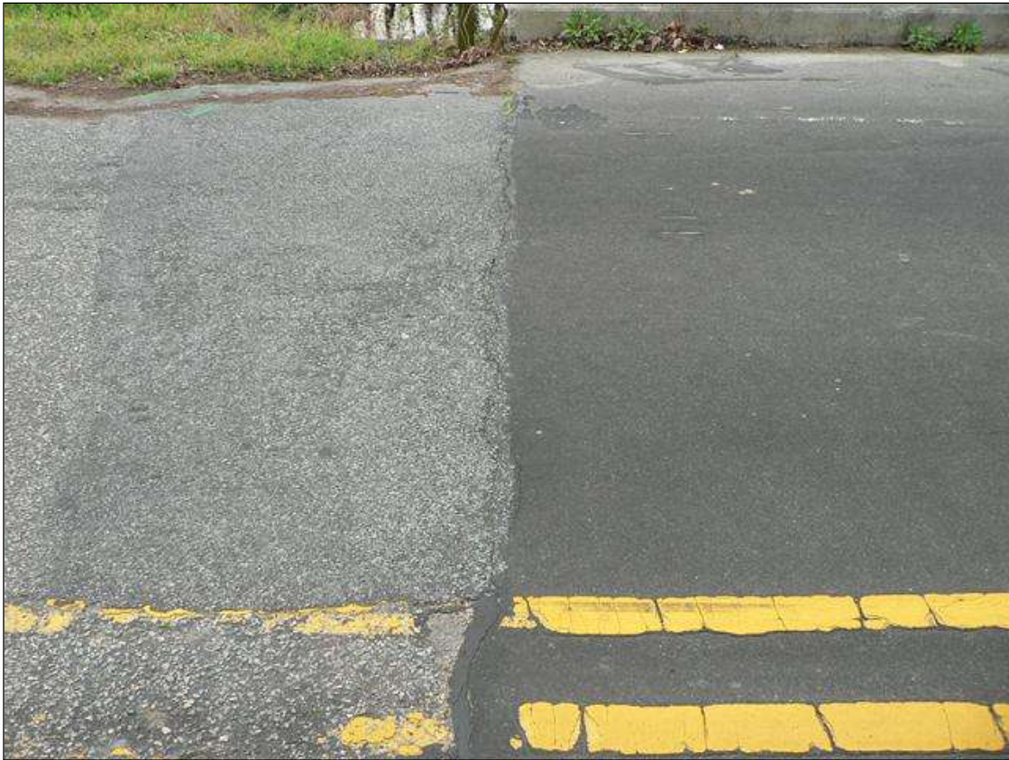
TRANSVERSE CRACK IN ASPHALT WEARING SURFACE ALONG END BENT 1 FILL FACE IN SOUTHBOUND LANE
