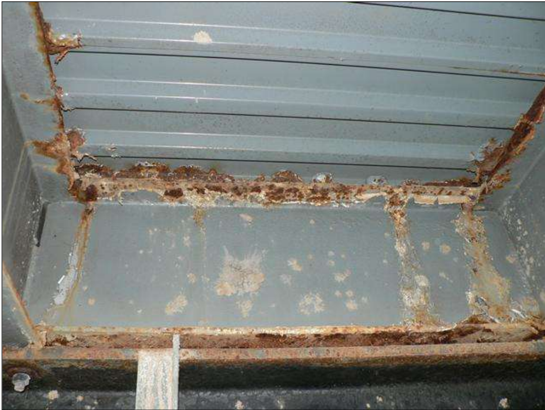
PAINT FLAKING AND PEELING AND SURFACE RUST ON END BENT 2 DIAPHRAGM IN BAY 4
