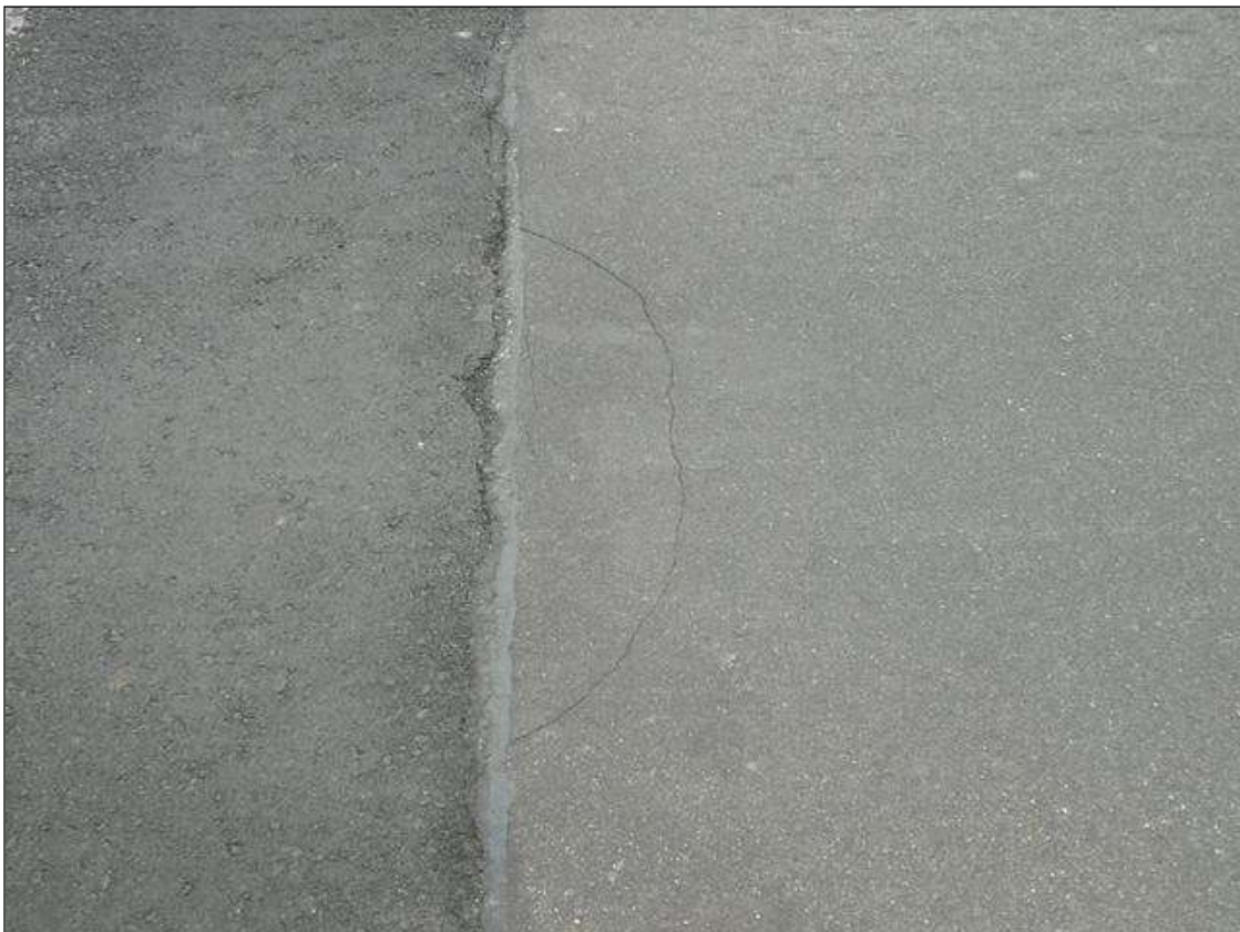
CRACK IN ASPHALT WEARING SURFACE IN NORTHBOUND LANE AT END BENT 1
