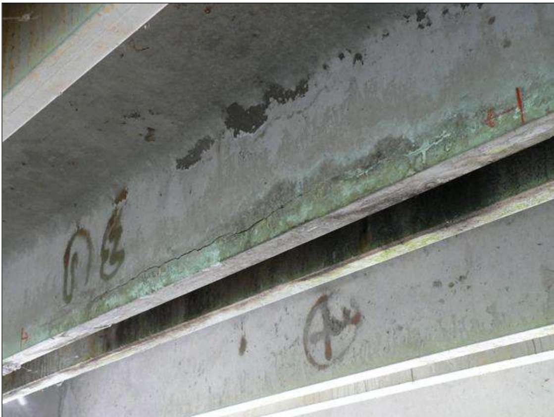
66" X 3" AREA OF DELAMINATION AND 1/8" HORIZONTAL CRACK IN LEG 2 OF CHANNEL 5 NEAR END BENT 2
