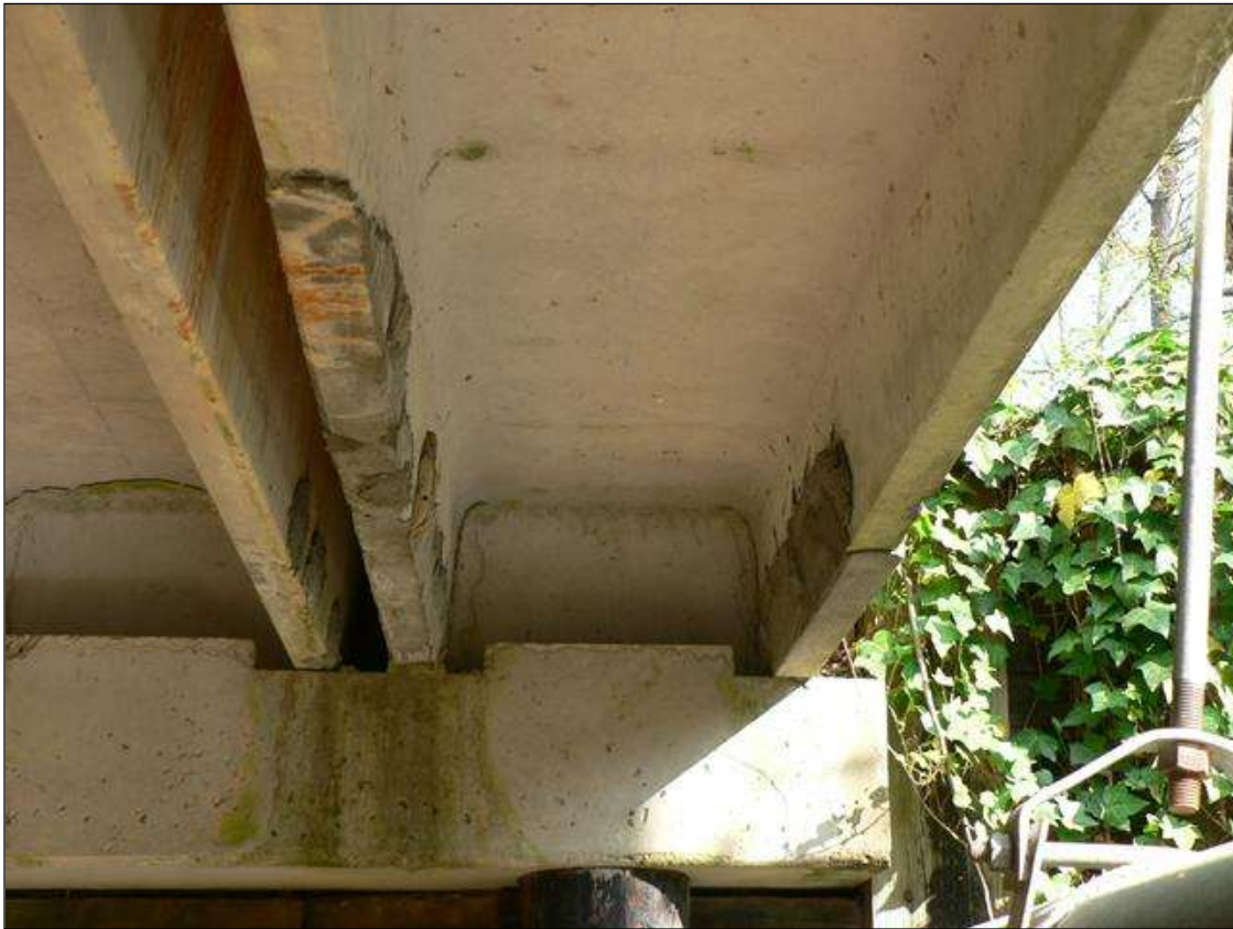
REPAIR TO LEGS 1 AND 2 OF CHANNEL 12 AT END BENT 2, LEG 2 OF CHANNEL 11 SIMILAR
