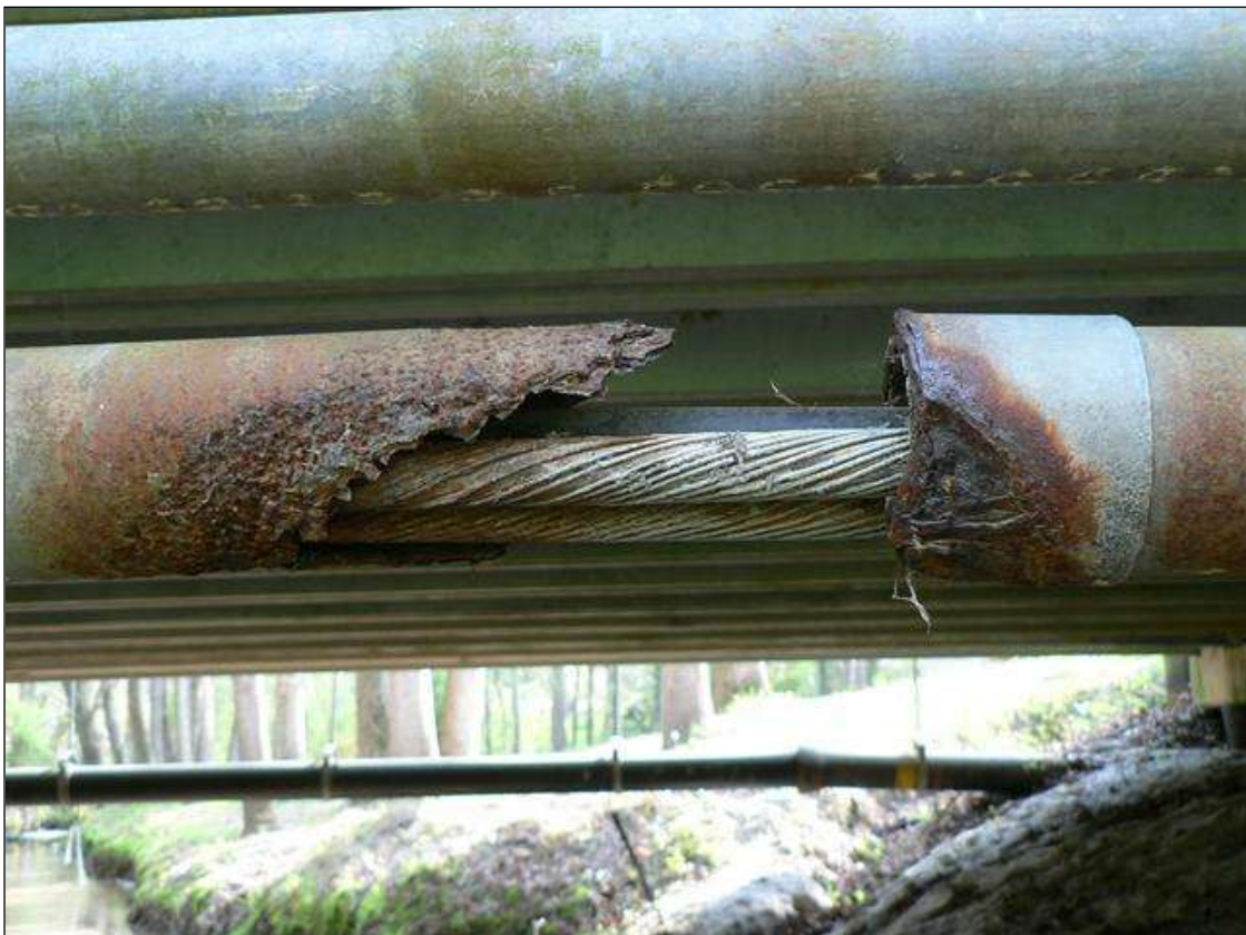
12" LONG SECTION OF DETERIORATION OF 4" DIAMETER STEEL UTILITY CONDUIT ON UPSTREAM SIDE
