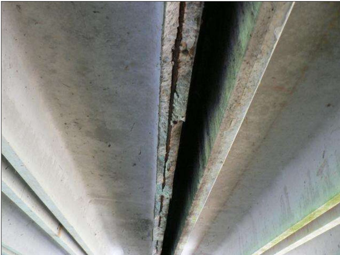
11' X 3" X 2" DEEP SPALL WITH EXPOSED STRAND IN LEG 2 OF CHANNEL 5 (PRIORITY MAINTENANCE)
