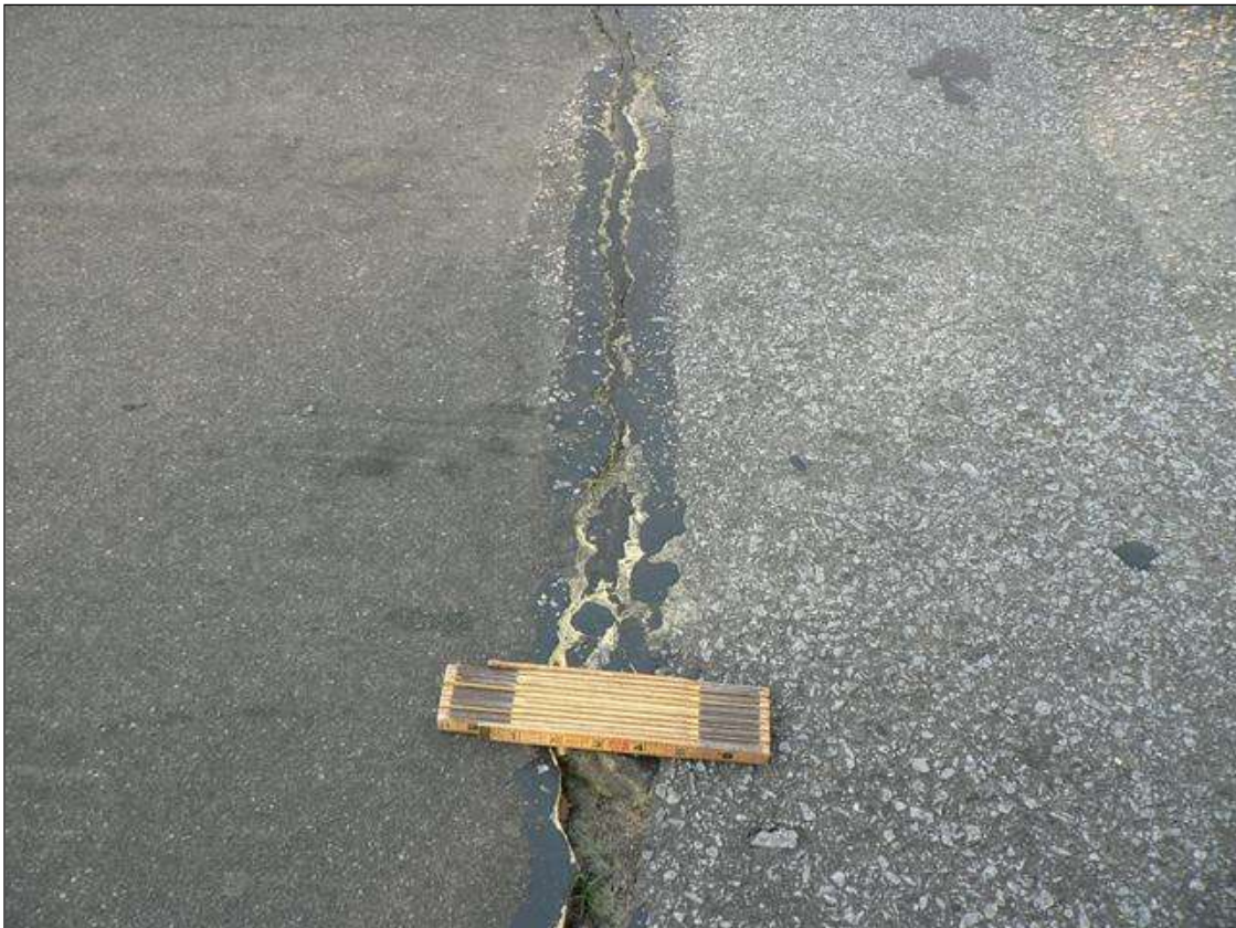
5" X 2" X 1" DEEP POT HOLE AND TRANSVERSE CRACK IN ASPHALT WEARING SURFACE ALONG END BENT 2 FILL FACE
