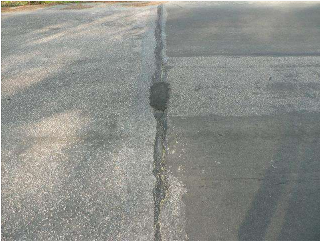
TRANSVERSE CRACKS IN ASPHALT WEARING SURFACE ALONG END BENT 1 FILL FACE
