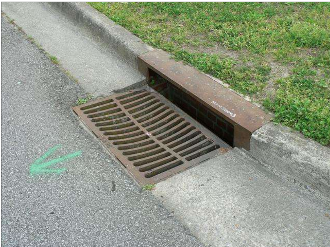
ROADWAY DRAIN ON WEST SIDE AT NORTH APPROACH, ROADWAY DRAIN ON EAST SIDE SIMILAR
