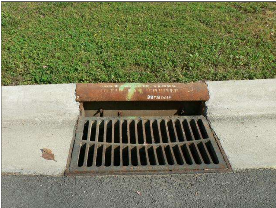
ROADWAY DRAIN ON NORTH SIDE AT WEST APPROACH, ROADWAY DRAIN ON SOUTH SIDE SIMILAR
