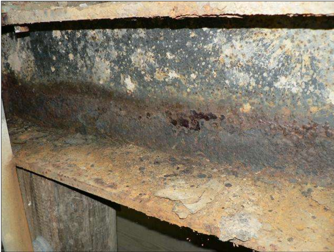
SCALING AND RUST PACKING IN END BENT 1 WEB BETWEEN PILES 4 AND 5
