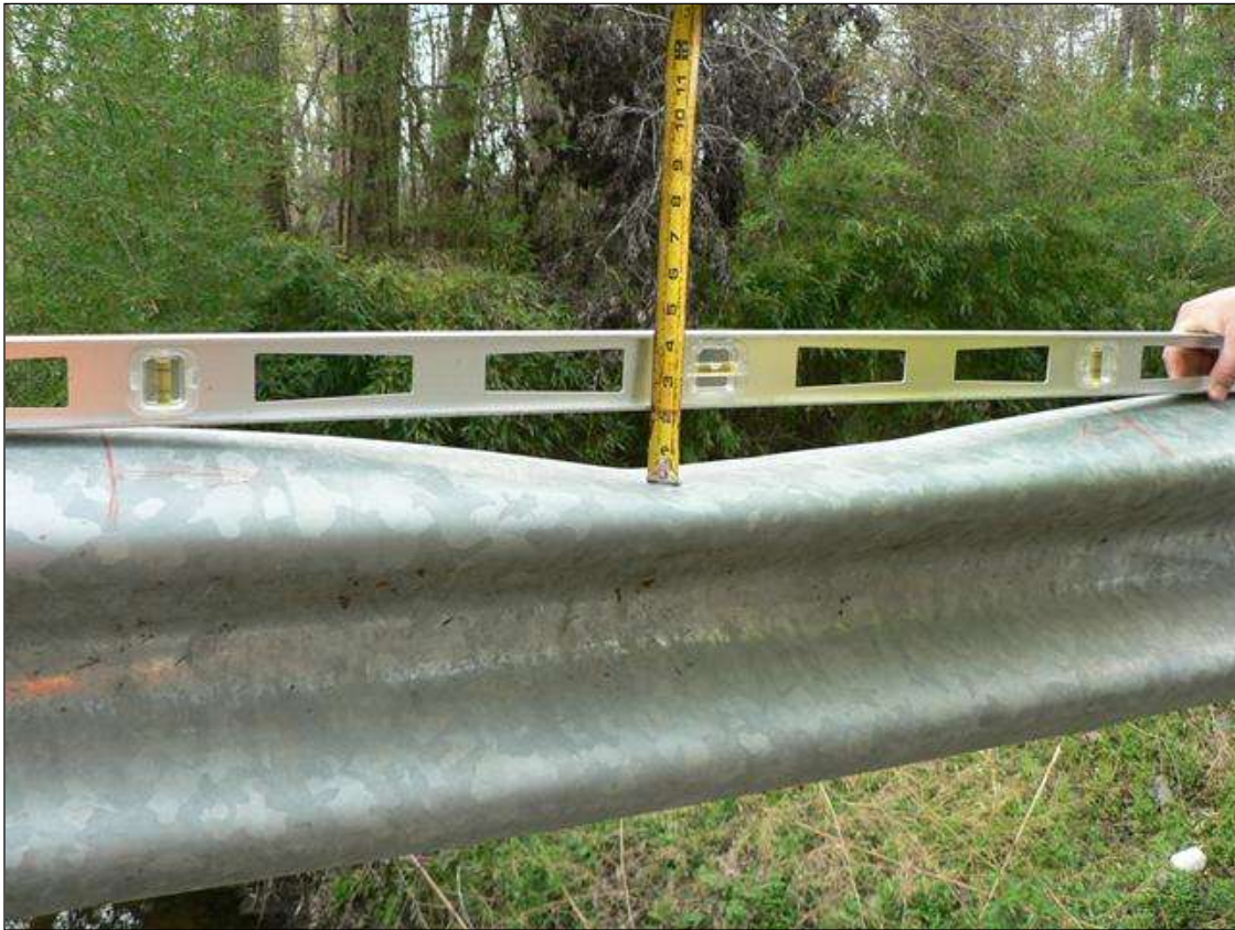
33" LONG X 2" DEEP AREA OF IMPACT DAMAGE TO UPSTREAM RAIL BETWEEN RAIL POSTS 2 AND 3
