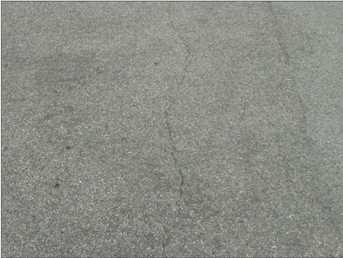
LONGITUDINAL CRACK IN ASPHALT WEARING SURFACE IN EASTBOUND LANE AT EAST APPROACH
