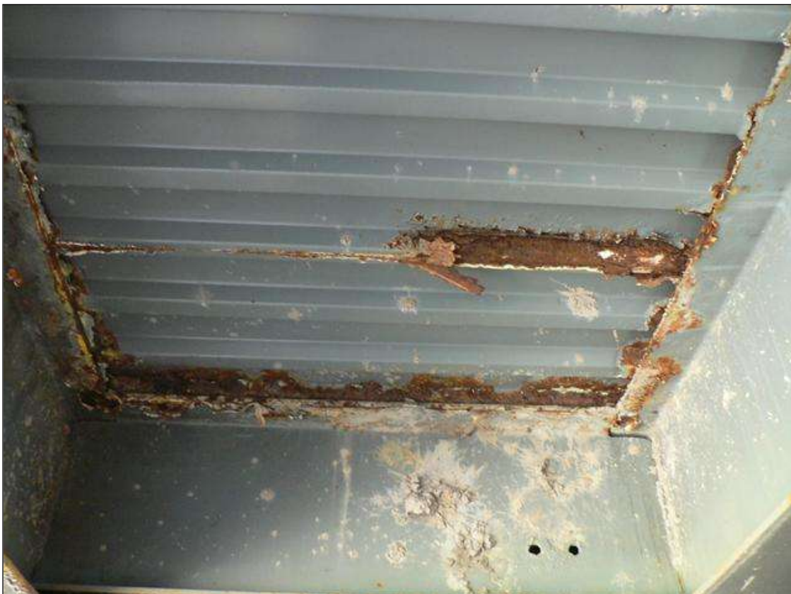
SCALING AND RUSTING IN BOTTOM OF SIP FORM IN BAY 1 AT END BENT 2
