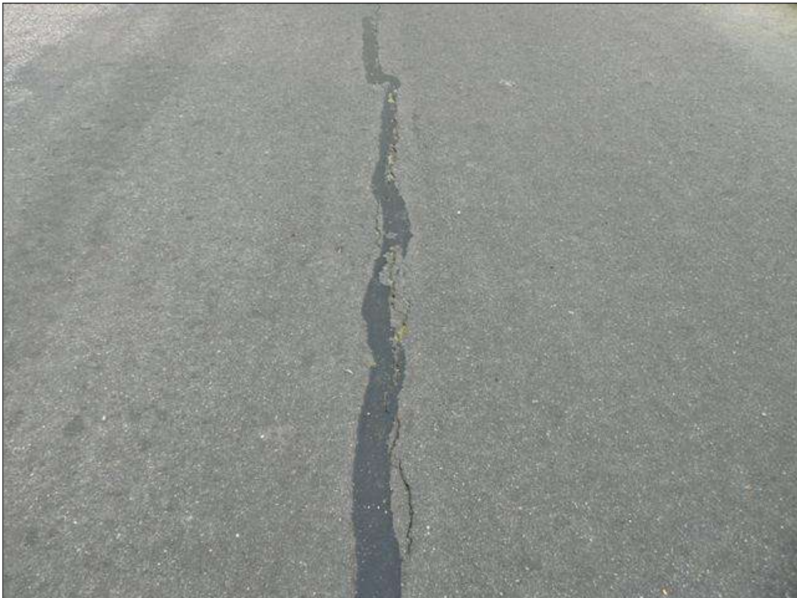
LONGITUDINAL CRACK IN ASPHALT WEARING SURFACE IN NORTHBOUND LANE
