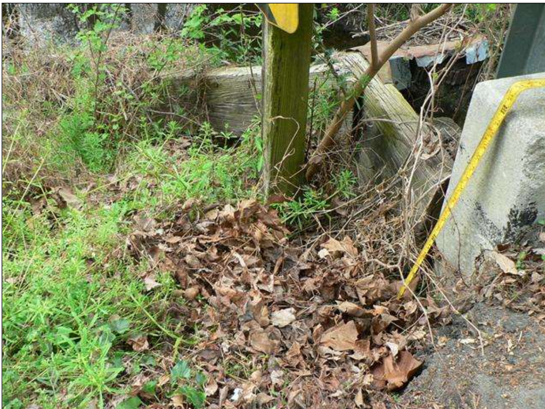
UP TO 12" DEEP SHOULDER EROSION BEHIND SOUTHWEST WINGWALL
