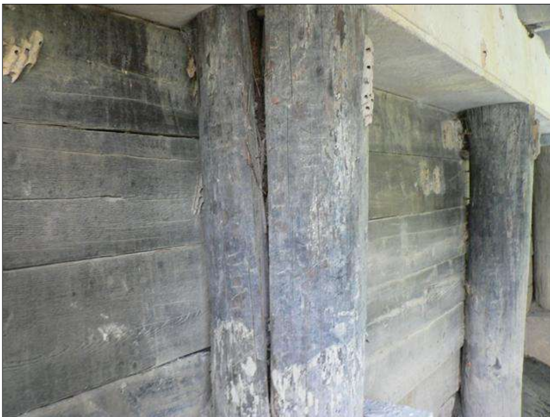
UP TO 1 1/2" WIDE X 4" DEEP SPLIT IN PILE 5 ON UPSTREAM AND DOWNSTREAM FACES FROM TOP OF CONCRETE COLLAR TO BOTTOM OF CAP AT END BENT 1
