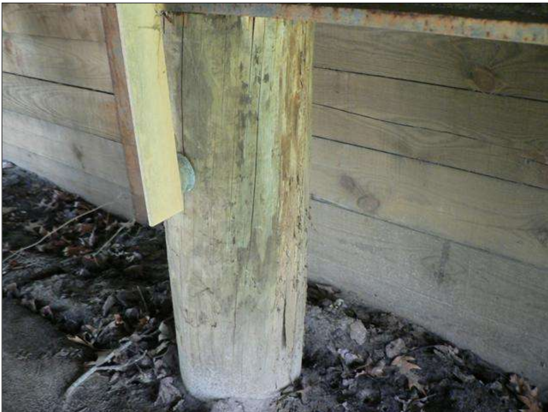
CHECKS AND SPLITS IN PILE 3 AT END BENT 1
