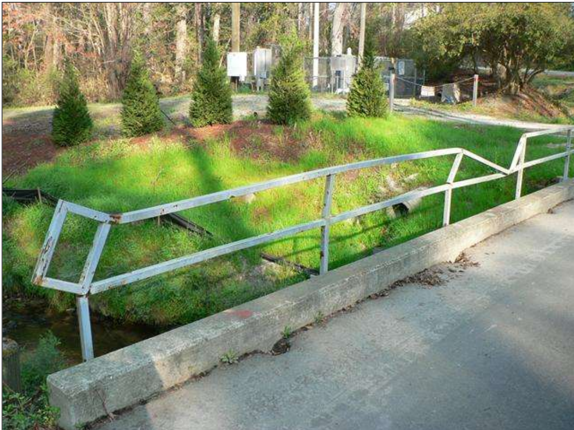
DAMAGE TO UPSTREAM RAIL
