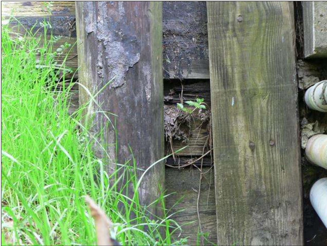
12" X 8" X 2" DEEP AREA OF DECAY IN NORTHWEST WINGWALL BEHIND WING PILE
