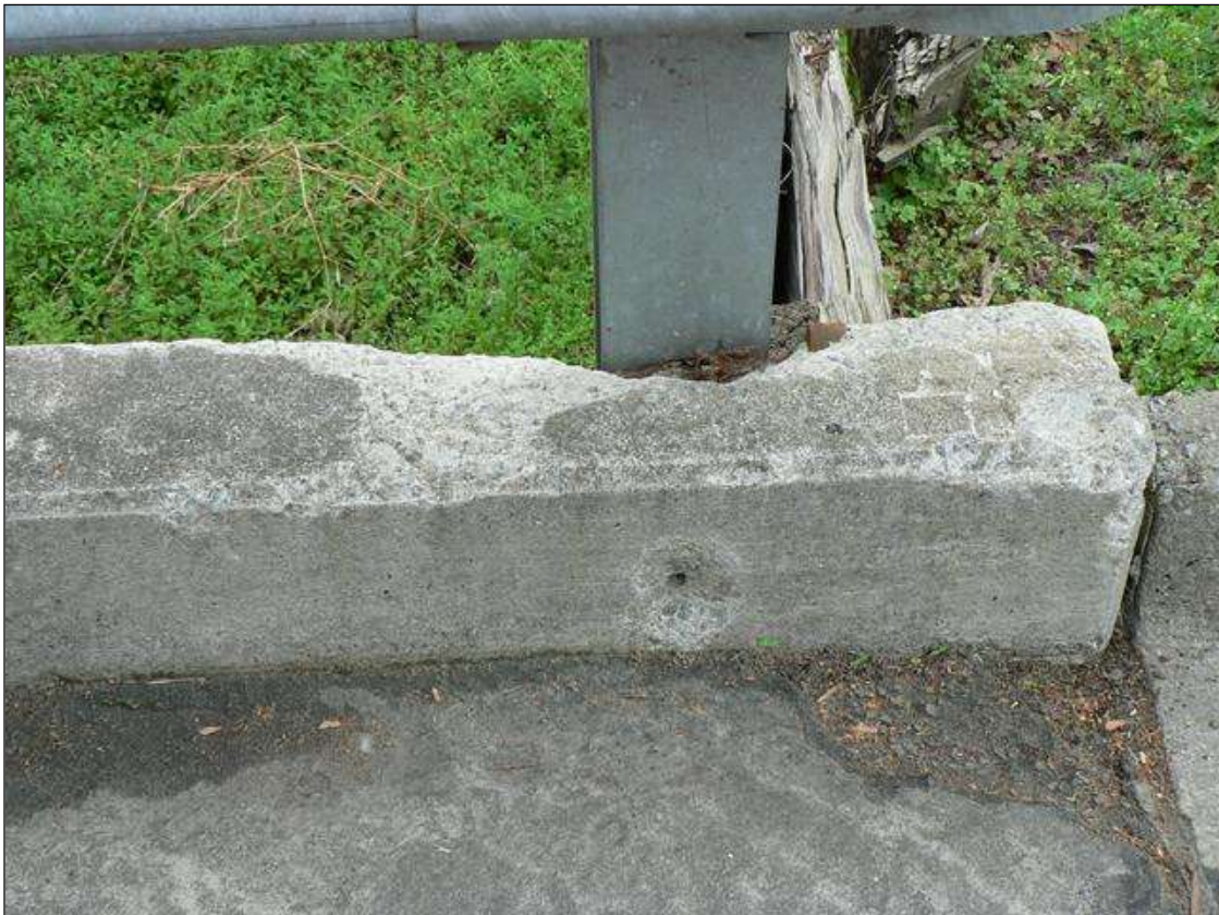
30" X 8" X 3" DEEP SPALL IN TOP AND 5" X 3" X 1/2" DEEP SPALL IN FACE OF UPSTREAM CURB AT NORTH END
