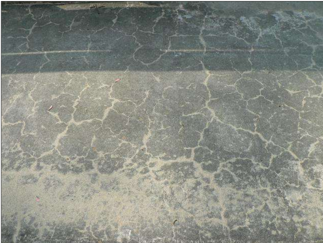
HAIRLINE MAP CRACKING WITH EFFLORESCENCE IN TOP OF UPSTREAM SIDEWALK NEAR WEST APPROACH
