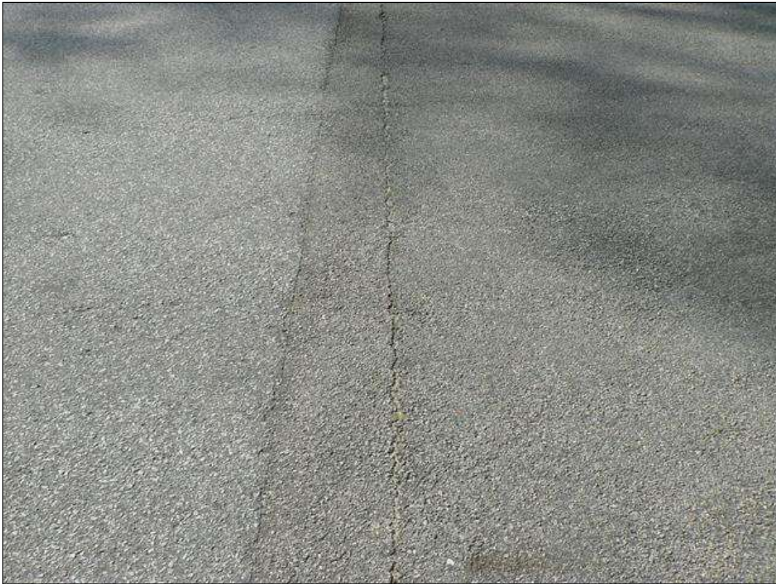
TRANSVERSE CRACK IN ASPHALT WEARING SURFACE ALONG END BENT 1 FILL FACE
