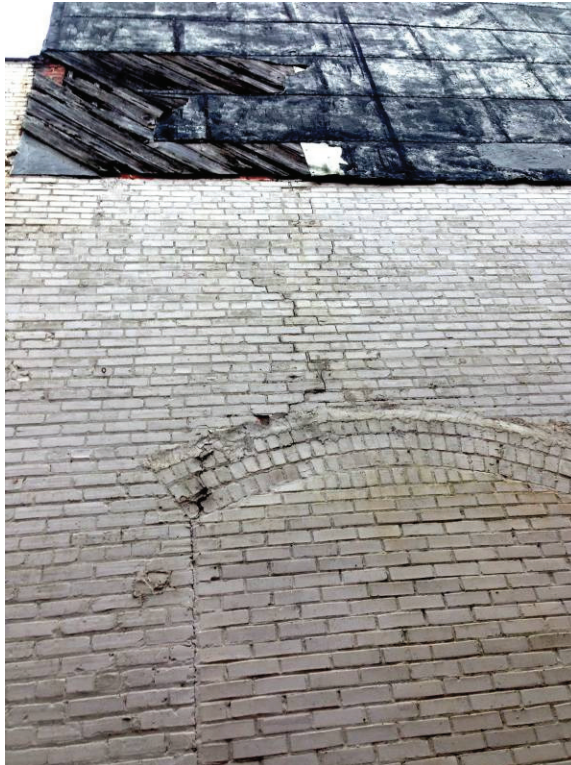
Photograph 6 – Sheathing Damage and Brick Crack at Left Side Fly Loft Wall
