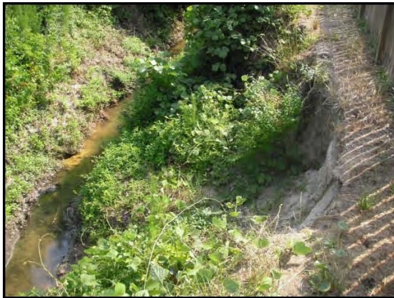
Picture 5-2. Severe bank erosion along landscaping fence
